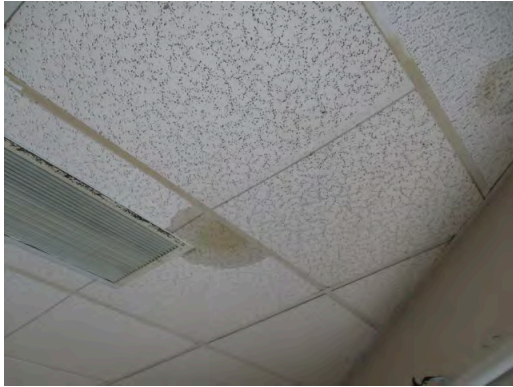
1982 addition classroom 26 ceiling staining
