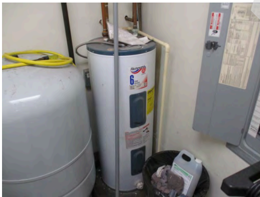
Water heater in 2000 addition utility room
