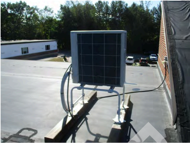
89. Condensing unit over 1962 section
