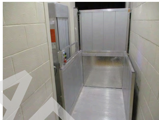
Wheelchair lift to stage/music room off gymnasium
