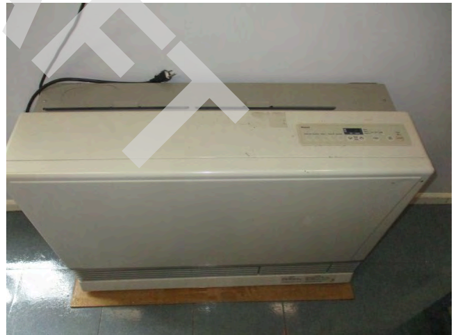
104. Typical Rinnai heater in 2000 addition
