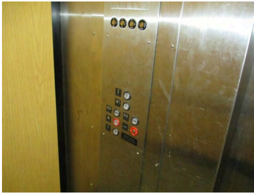
Elevator cab controls
