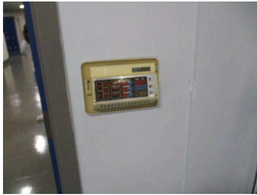
Thermostat in 1982 classroom
