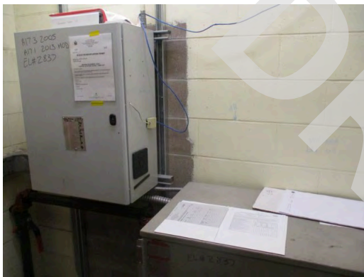
Elevator hydraulic unit
