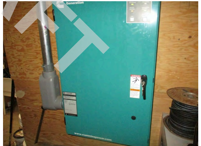
116. Generator transfer switch in 1982 boiler room
