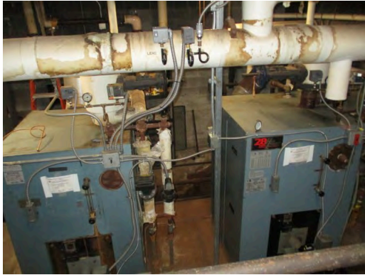
Boiler room in 1956 section
