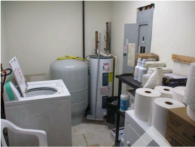
181. Utility room in 2000 addition
