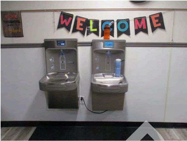
109. Water bottle fillers in 2000 addition corridor
