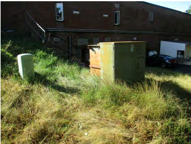
119. Pad-mount transformer north of 1982 section
