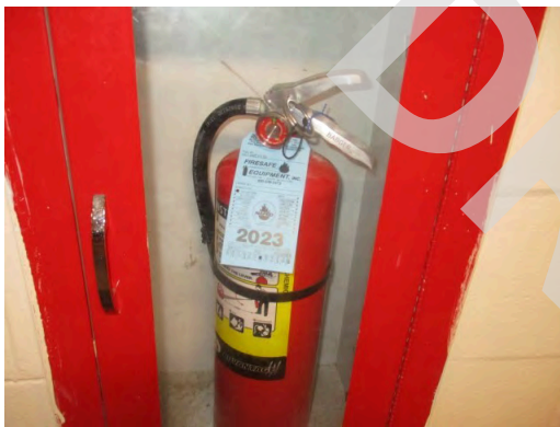
Typical fire extinguisher in corridor
