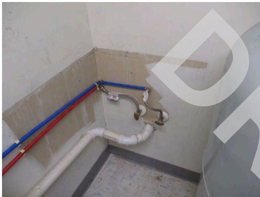
Damaged sheetrock in 2000 addition utility room
