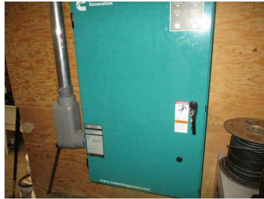
Generator transfer switch in 1982 boiler room
