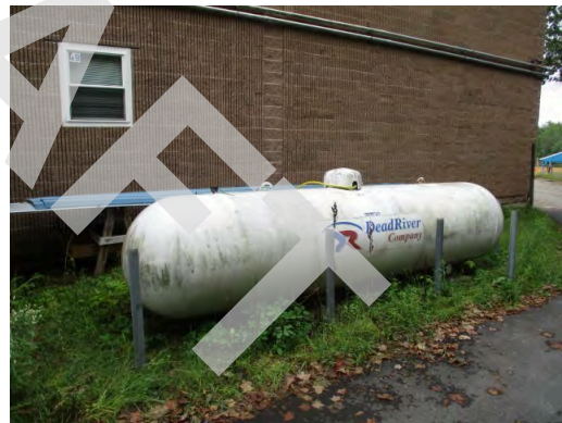
Propane AST behind gymnasium
