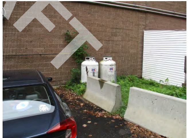
100. Propane cylinders behind kitchen
