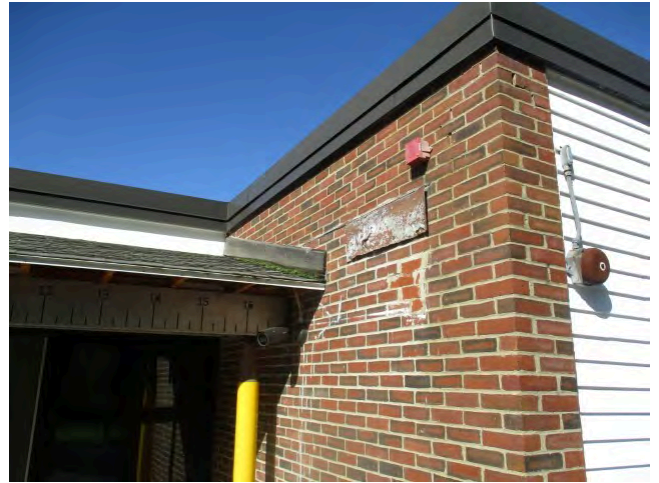
10. Cracking in facade on north side of east entrance
