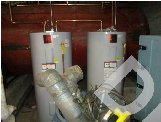
Domestic water heaters in 1982 boiler room
