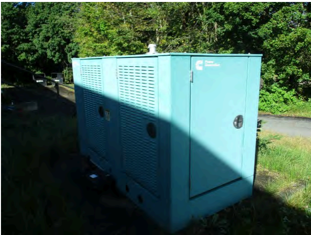
115. Emergency generator north of 1982 section
