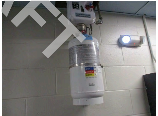
124. Ansul system in kitchen
