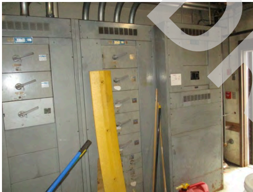
Main electrical panels in 1982 electrical room
