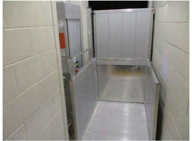
130. Wheelchair lift to stage/music room off gymnasium
