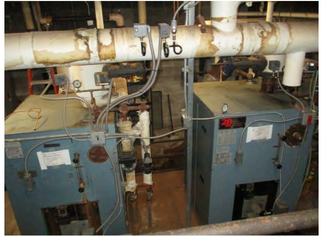
86. Boiler room in 1956 section
