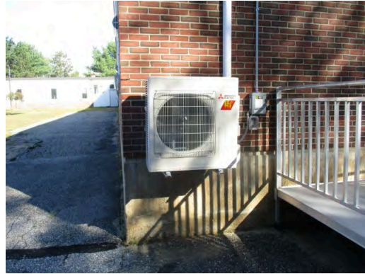
Condensing unit on south side of 1956 section
