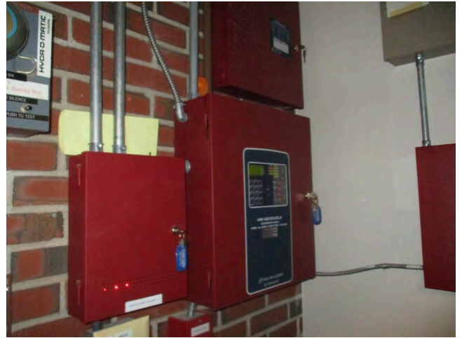
122. Fire alarm panel in main office
