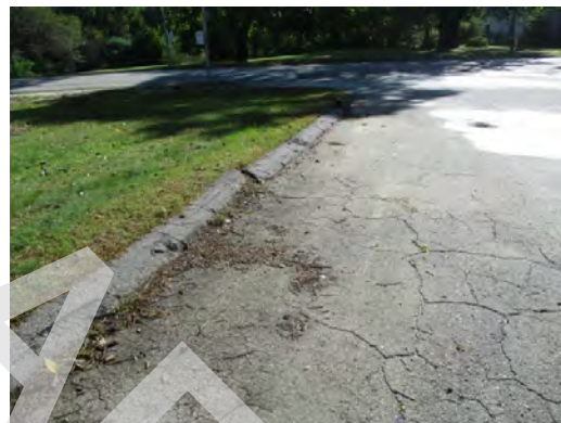
Damaged curbing east of building
