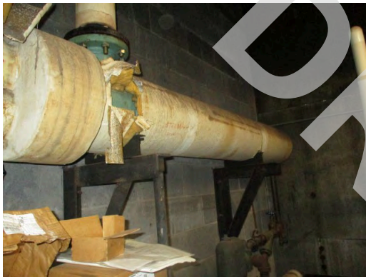
Damaged heat exchanger in 1956 boiler room
