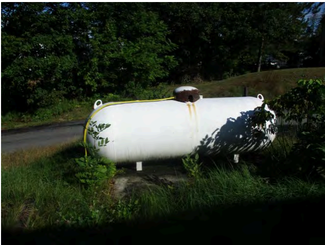
99. Propane AST for emergency generator north of 1982 section
