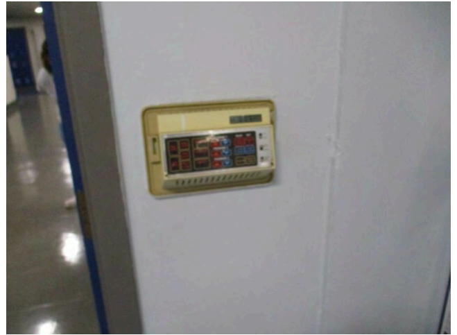
102. Thermostat in 1982 classroom
