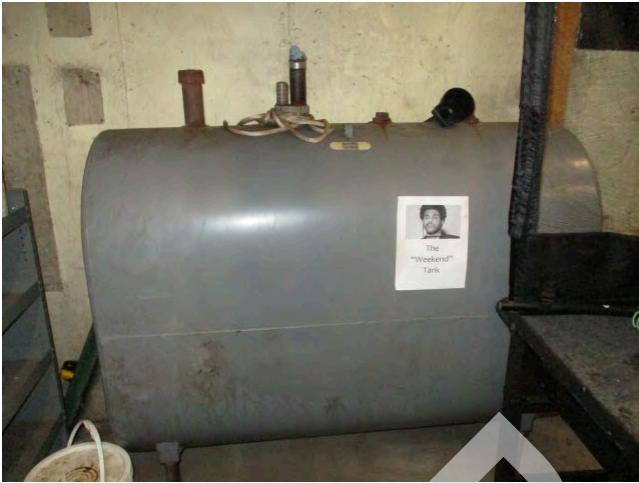
97. Old heating oil AST in 1982 boiler room (not in service)
