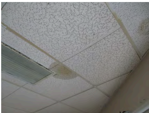
1982 addition classroom 26 ceiling staining
