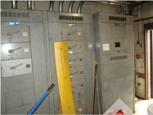
117. Main electrical panels in 1982 electrical room
