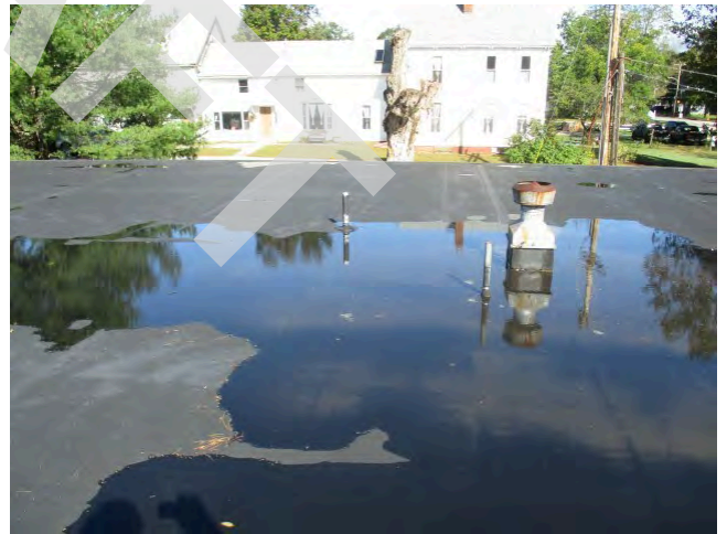
60. Roof ponding over 1956 section
