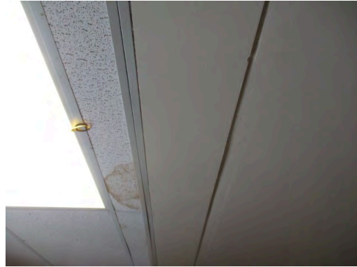
Staining at ceiling junction between 1982 section and 2002 addition
