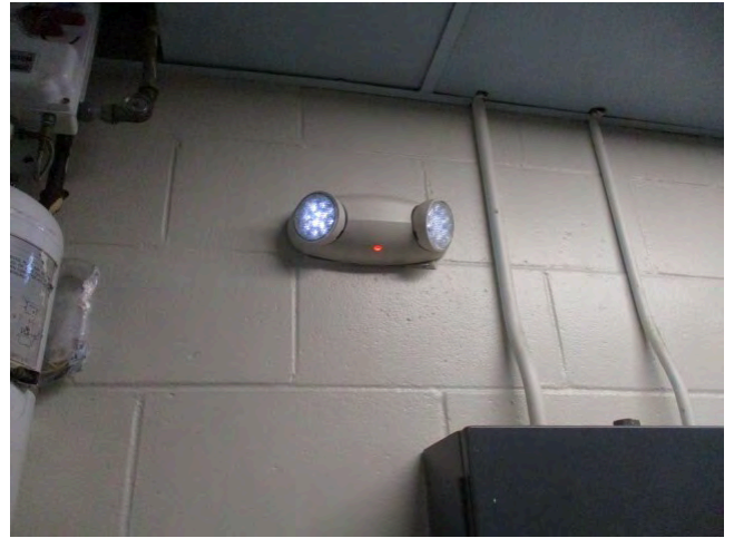
118. Malfunctioning emergency lights in kitchen
