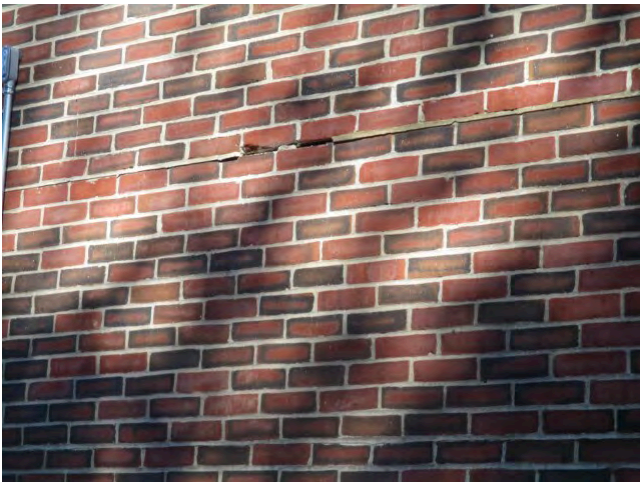
7. Cracking in brick facade in 1956 section
