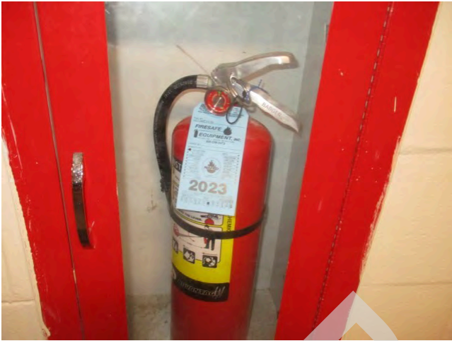
125. Typical fire extinguisher in corridor
