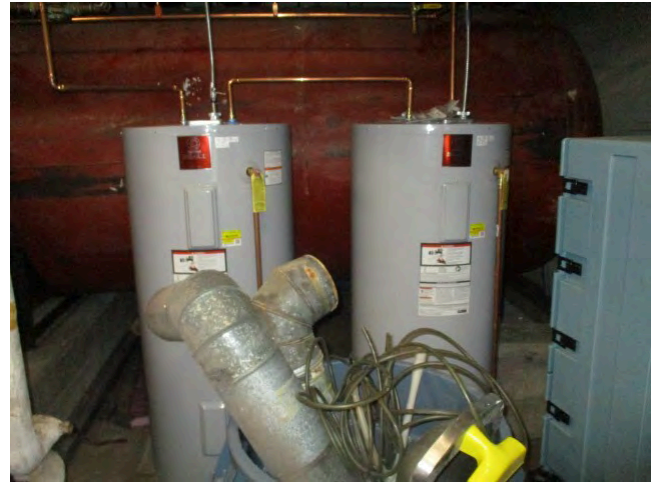
106. Domestic water heaters in 1982 boiler room
