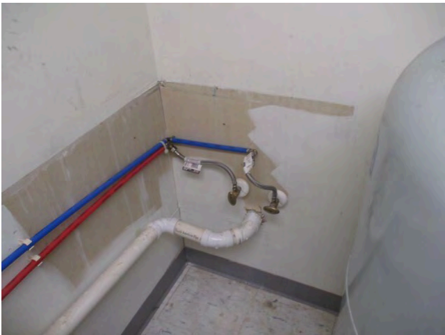
183. Damaged sheetrock in 2000 addition utility room
