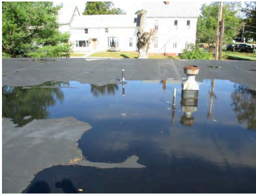
Roof ponding over 1956 section
