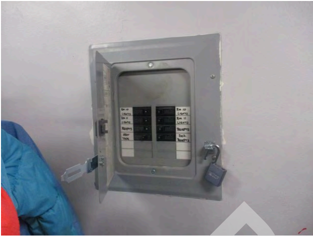
121. Typical subpanel in classroom 34
