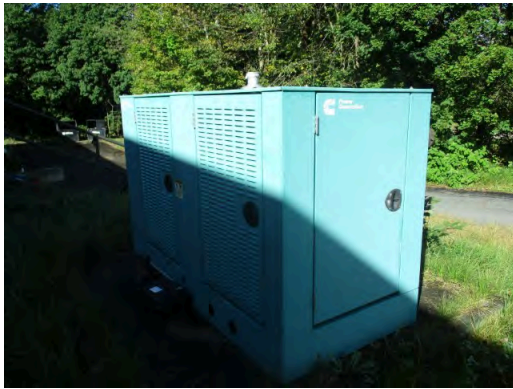
Emergency generator north of 1982 section
