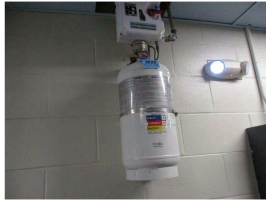
Ansul system in kitchen
