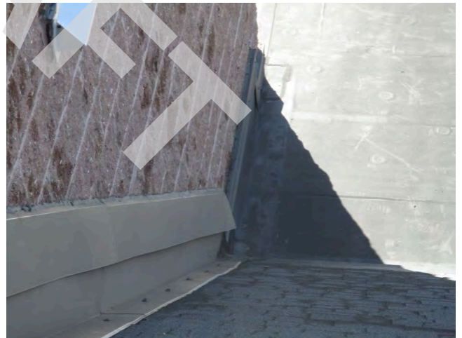
80. Roof junction over problem area at 1982 section and 2000 connector
