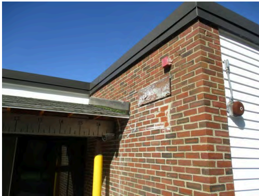
Cracking in facade on north side of east entrance
