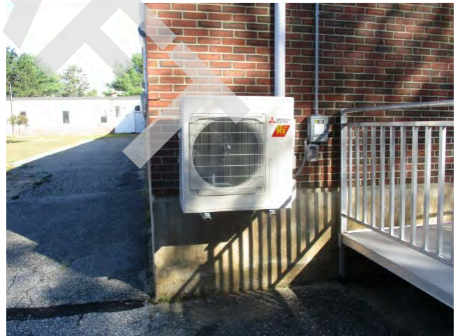
88. Condensing unit on south side of 1956 section
