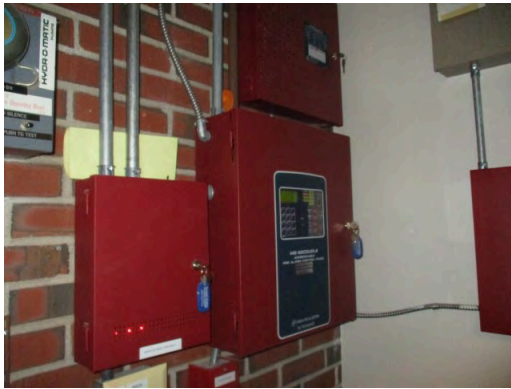
Fire alarm panel in main office
