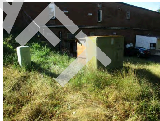
Pad-mount transformer north of 1982 section
