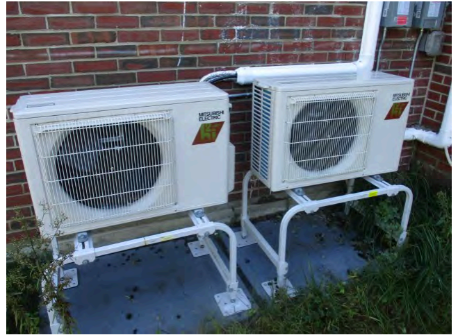
90. Condensing units on north side of 1982 section
