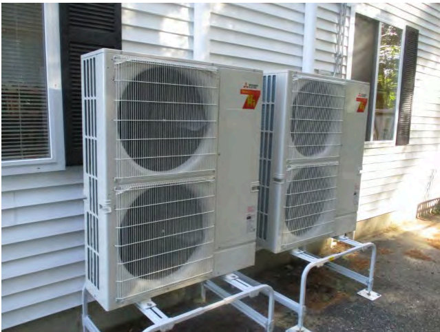
91. Condensing units on south end of 2000 addition
