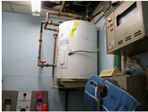
Water heater in janitor closet near gymnasium
