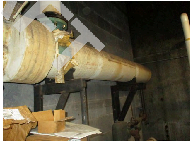
92. Damaged heat exchanger in 1956 boiler room
