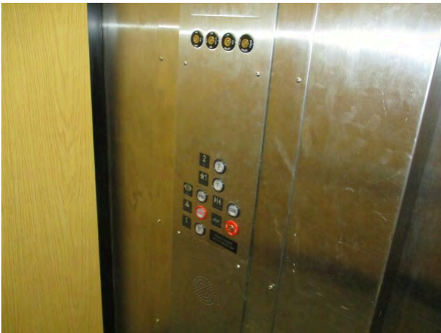
127. Elevator cab controls
