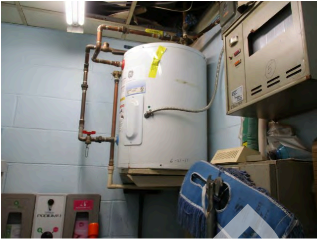
113. Water heater in janitor closet near gymnasium
