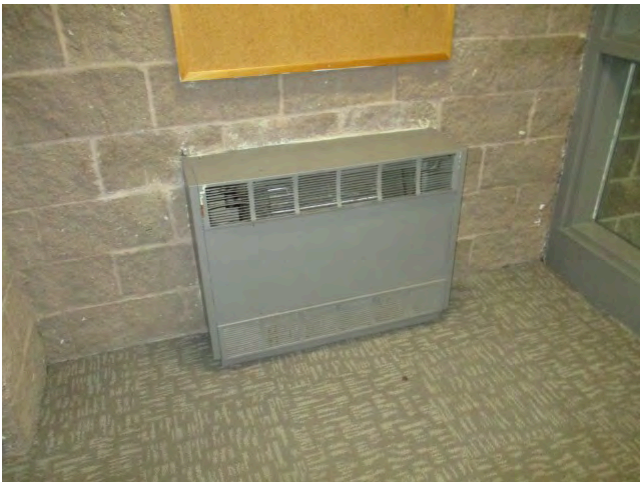
95. Hydronic radiator in corridor near gymnasium
