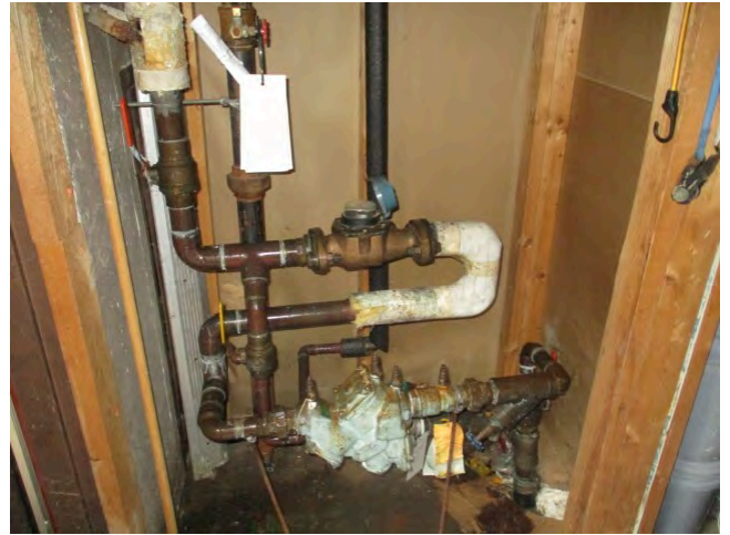
110. Water entrance near gymnasium
