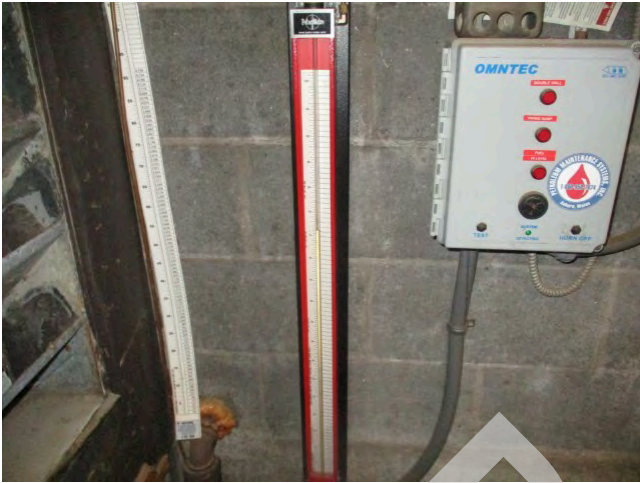
93. Heating oil UST level gauge in 1956 boiler room
