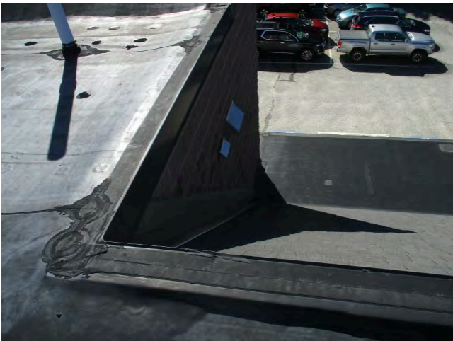
79. Roof section over problem area at 1982 section and 2000 connector
