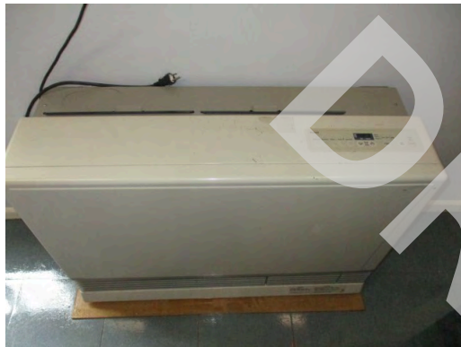
Typical Rinnai heater in 2000 addition
