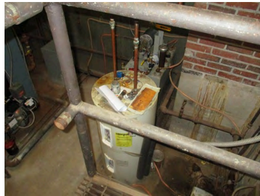
Water heater in 1956 boiler room
