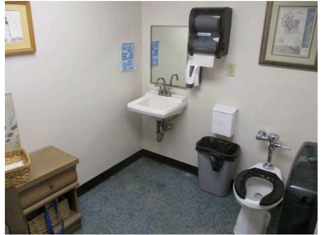
178. Staff restroom in 2000 addition
