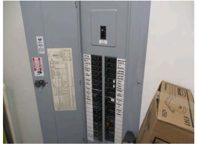
114. Electrical panel in 2000 utility room
