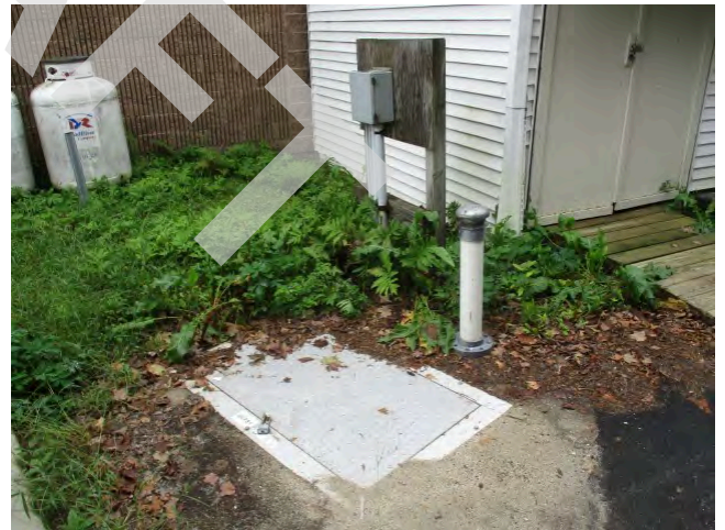
108. Sewer lift station behind gymnasium
