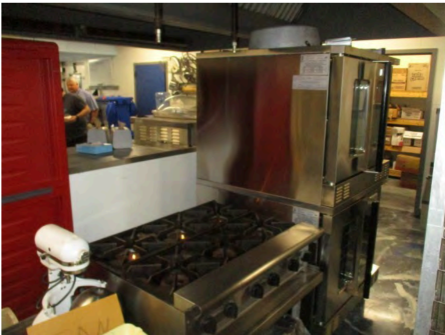
123. Ansul system in kitchen
