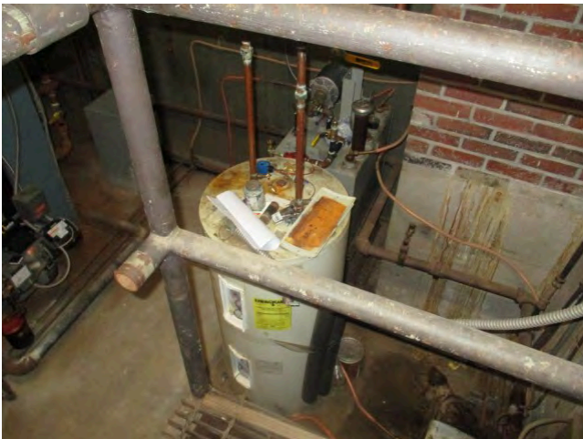
111. Water heater in 1956 boiler room
