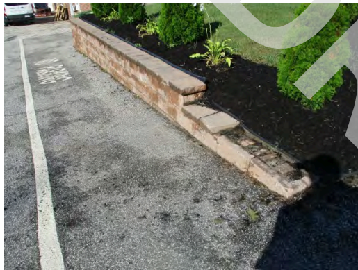
Retaining wall near main entrance showing missing blocks
