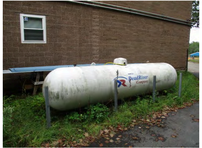
98. Propane AST behind gymnasium
