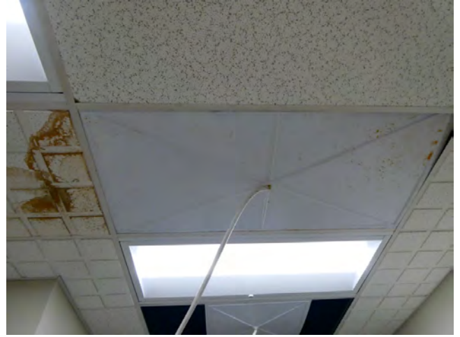
118. Interiors - Active roof leak at south portion
