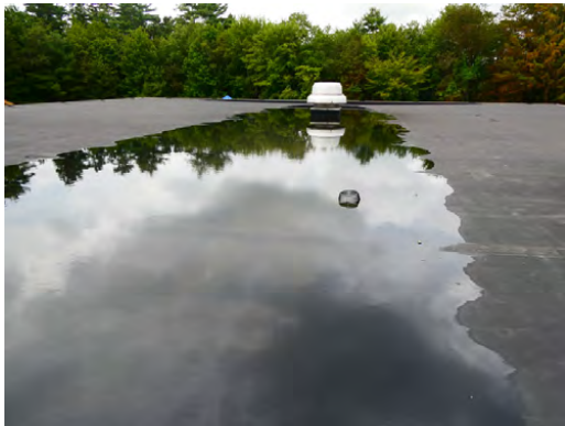
Roof - Standing water at northeast roof surface
