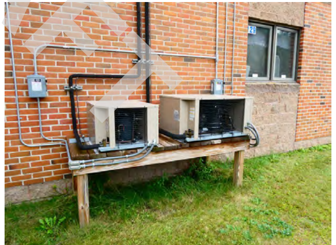
88. MEP - Kitchen refrigeration equipment
