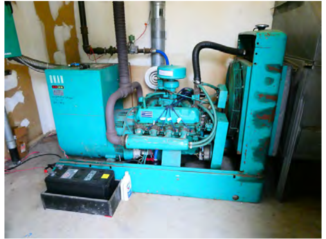
94. MEP - Natural gas-fired emergency generator
