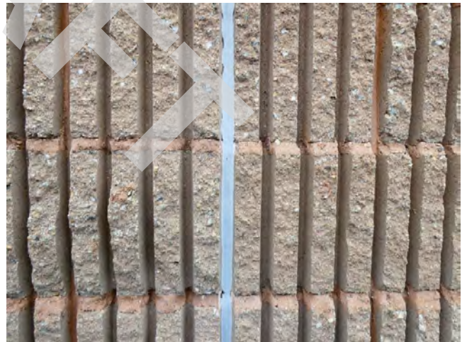
40. Exterior - Vertical sealant condition
