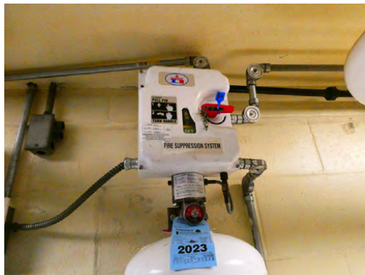
FLS - ANSUL fire suppression system tank
