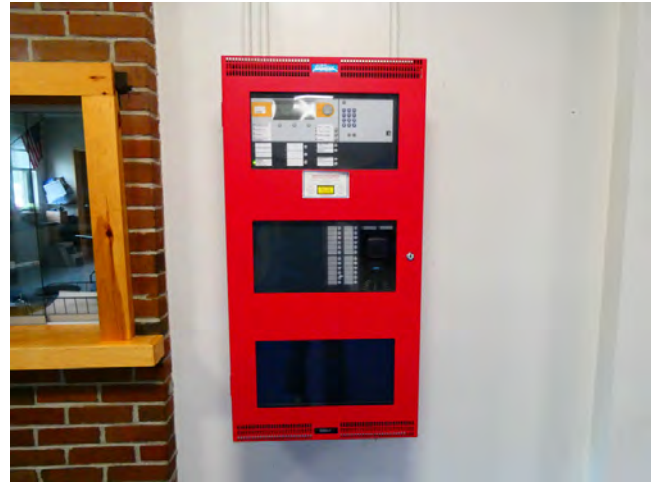
106. FLS - Main fire alarm control panel
