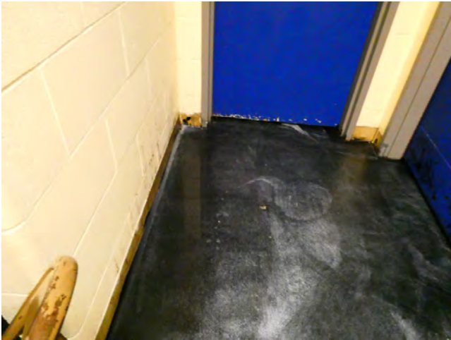
119. Interiors - Isolated leak at the kitchen bathroom area
