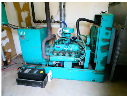
MEP - Natural gas-fired emergency generator
