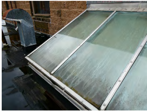
Roof - Skylight glazing with fogging condition
