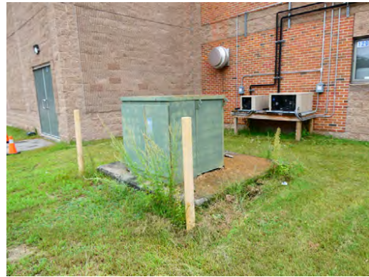
MEP - Pad mounted electrical transformer
