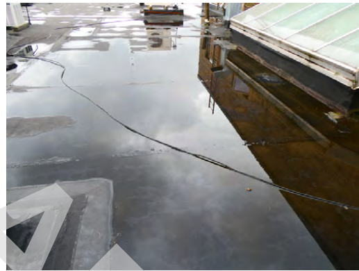
Roof - Standing water at central roof surface
