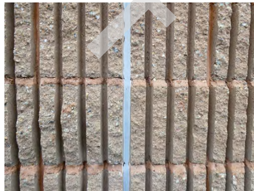
Exterior - Vertical sealant condition
