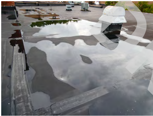
Roof - Standing water at central roof surface
