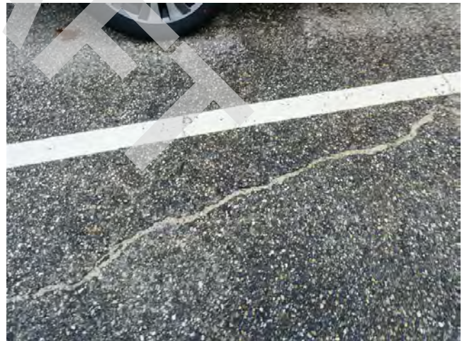
8. Site - Longitudinal cracking along south parking area
