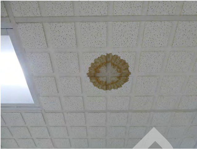
121. Interiors - Moisture stained ceiling tiles at south portion
