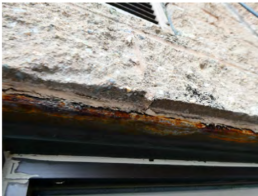
Exterior - Corrosion at steel lintels at roofline and deteriorated sealants
