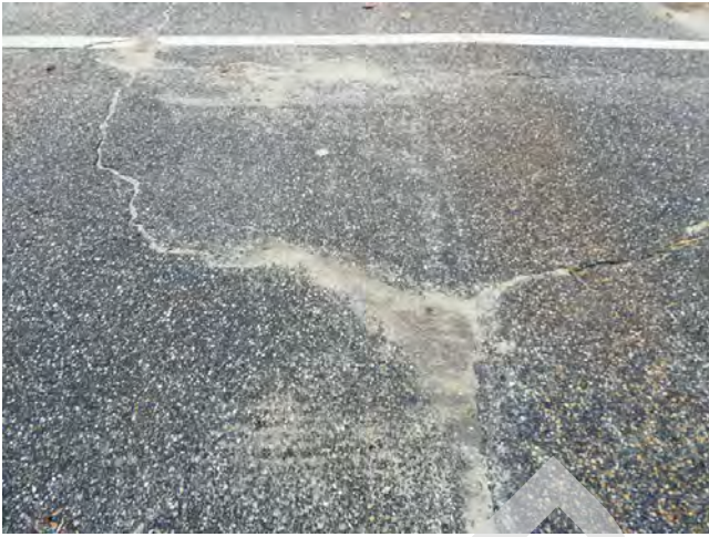
9. Site - Longitudinal cracking along south parking area
