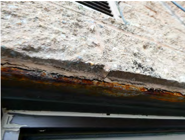
39. Exterior - Surface corrosion along steel lintels at roofline
