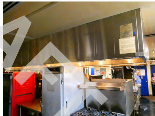
Interiors - Range hood with fire suppression system
