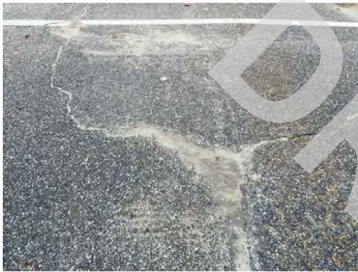
Site - Longitudinal cracking along south parking area
