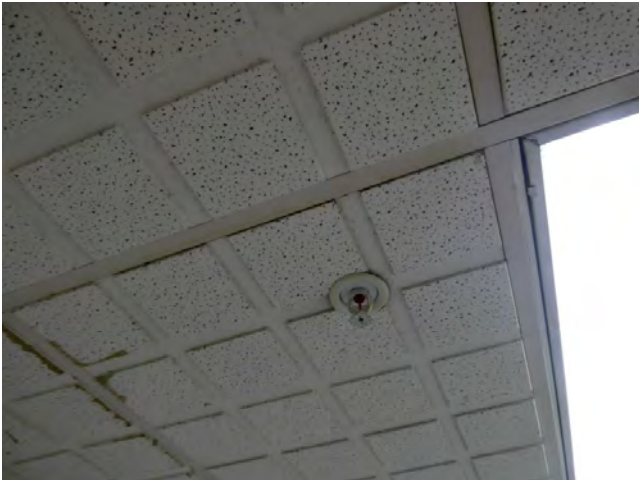
103. FLS - Fire suppression system sprinkler head
