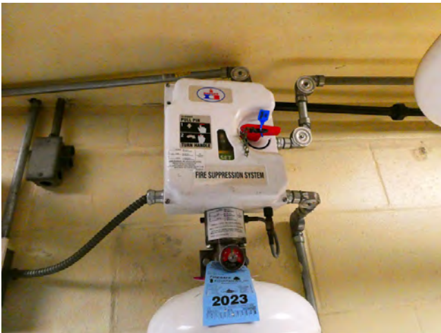
99. FLS - ANSUL fire suppression system tank
