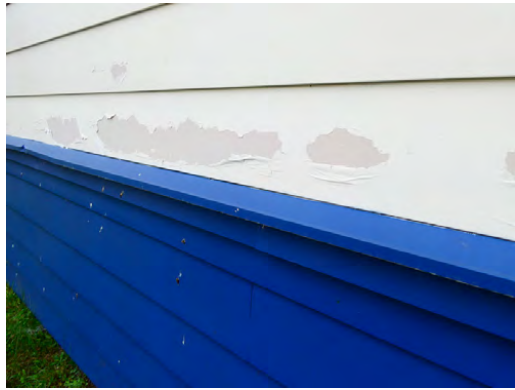
Exterior - Worn paint finish along north elevation
