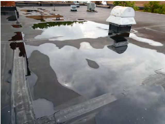
51. Roof - Standing water at central roof surface
