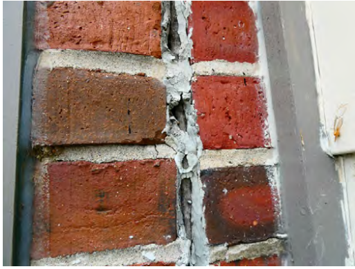
Exterior - Deteriorated vertical sealants along north elevation
