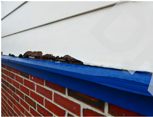
Exterior - Isolated deteriorated wood fiber siding (west elevation)
