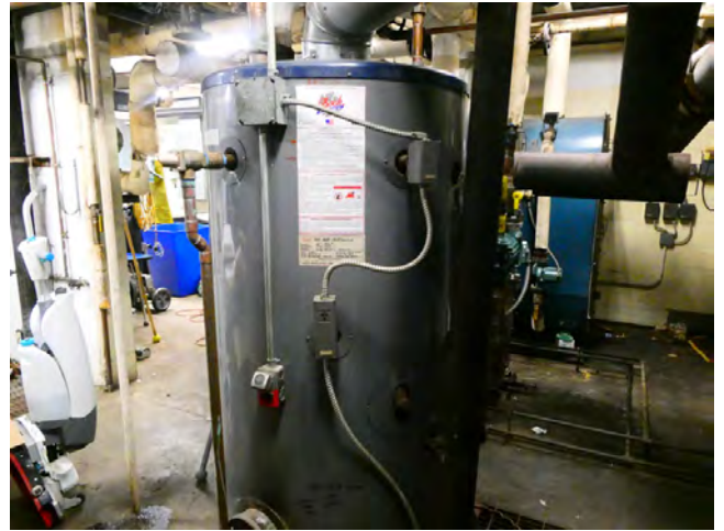
78. MEP - Gas fired domestic water heater
