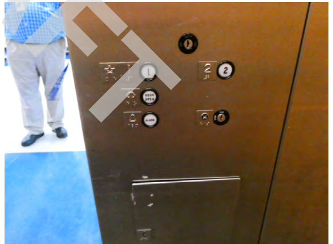
96. Vertical Transportation - Elevator controls
