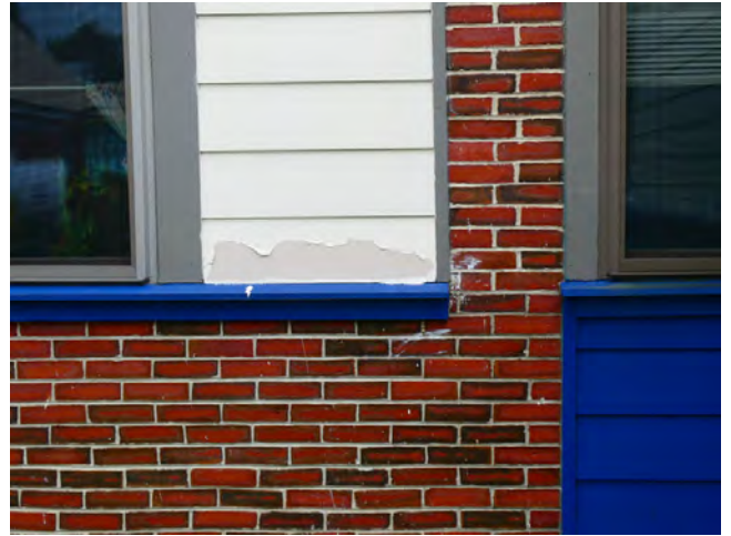
42. Exterior - Worn paint finish along north elevation
