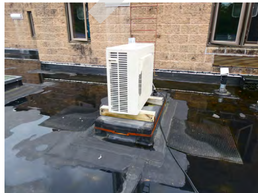
MEP - Roof mounted condenser for mini split system
