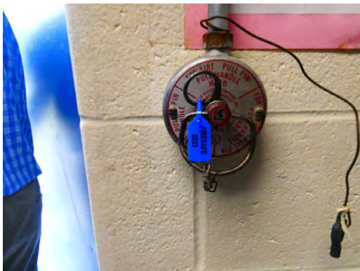
FLS - Kitchen ANSUL fire pull station
