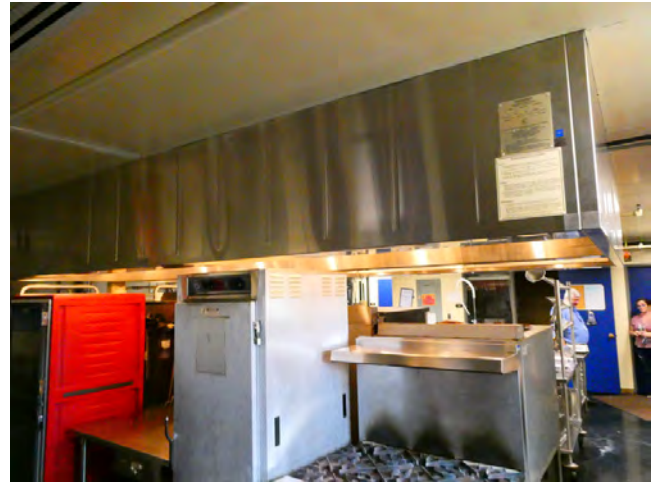
70. Interiors - Range hood with fire suppression system
