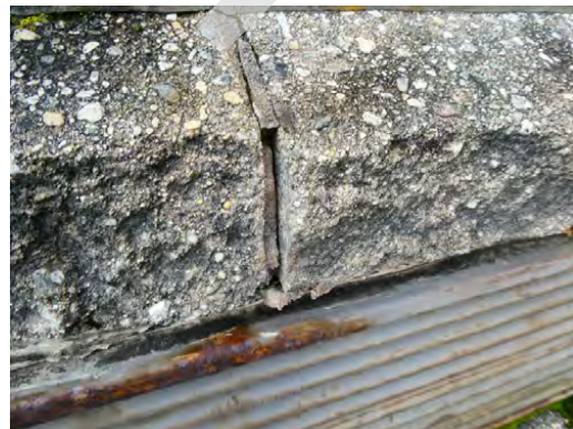
Exterior - Deteriorated mortar joints at CMU along roofline
