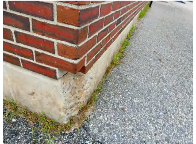
22. Structure - Damaged section of exposed concrete slab and missing brick
