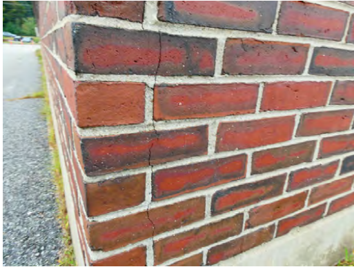
Structure - Vertical cracking along brick facade (northeast corner)
