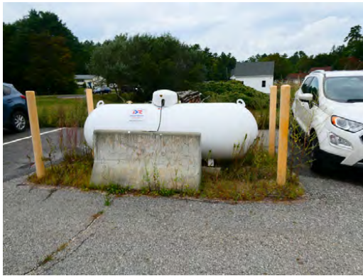
MEP - Onsite propane tank
