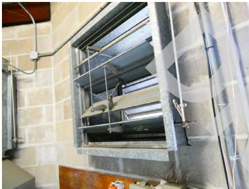
MEP - Natural ventilation exhaust in generator room
