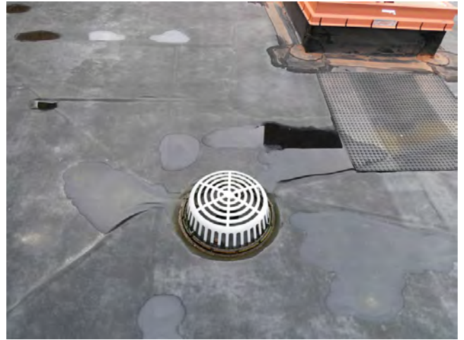
50. Roof - Internal roof drain and cover type
