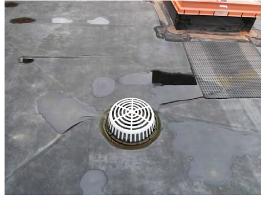
Roof - Internal roof drain and cover type
