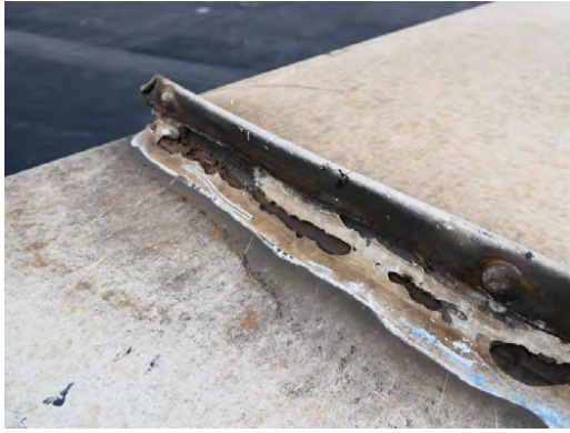
Roof - Deteriorated sealants at parapet wall flashing (central roof)
