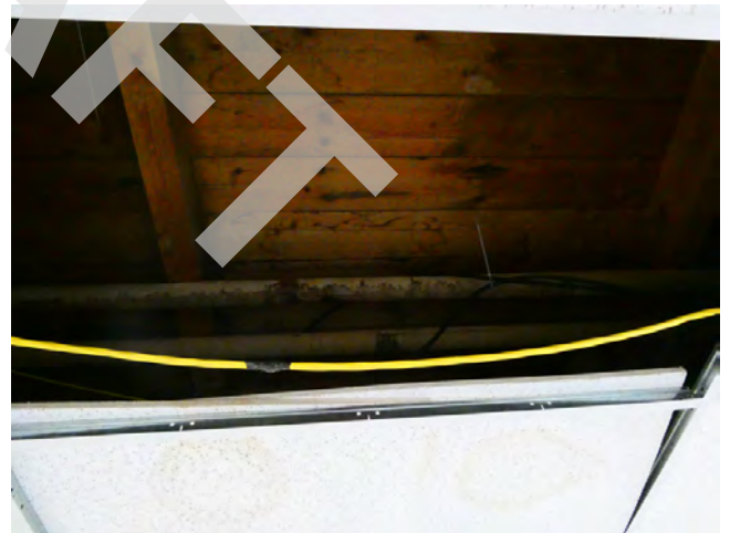
112. Interiors - Active roof leak at north corridor
