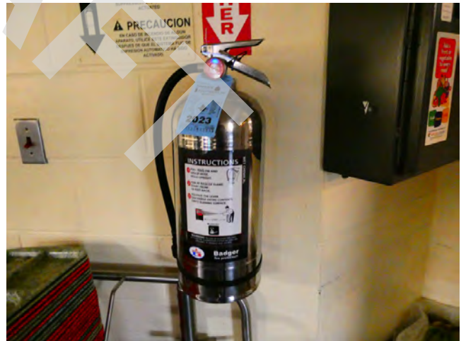
100. FLS - Chemical fire suppression extinguisher
