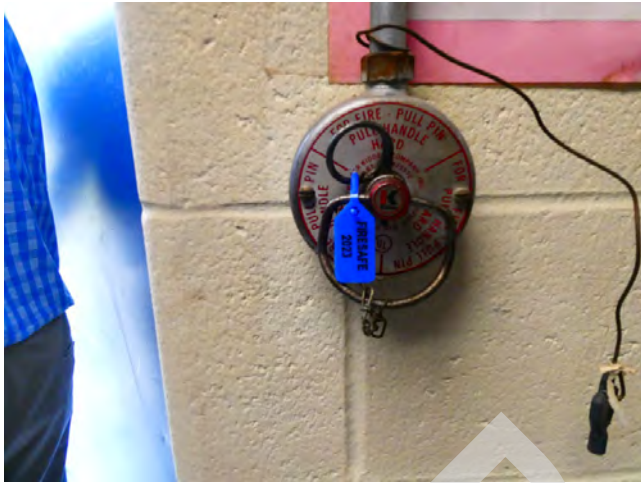
105. FLS - Kitchen ANSUL fire pull station
