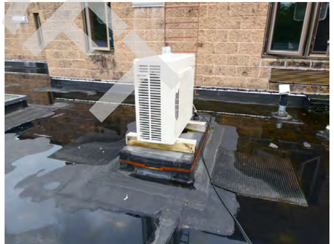
84. MEP - Roof mounted condenser for mini split system
