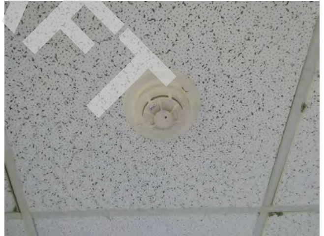
104. FLS - Hardwired ceiling mounted smoke detectors
