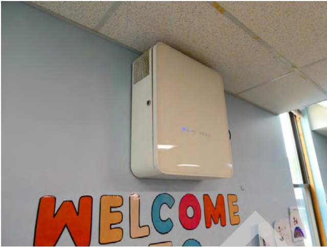
89. MEP - Ductless ERV system in classrooms
