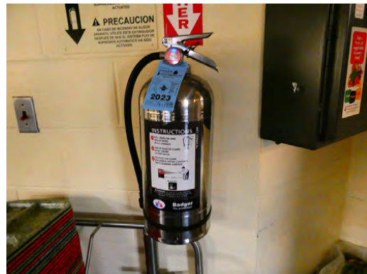
FLS - Chemical fire suppression extinguisher
