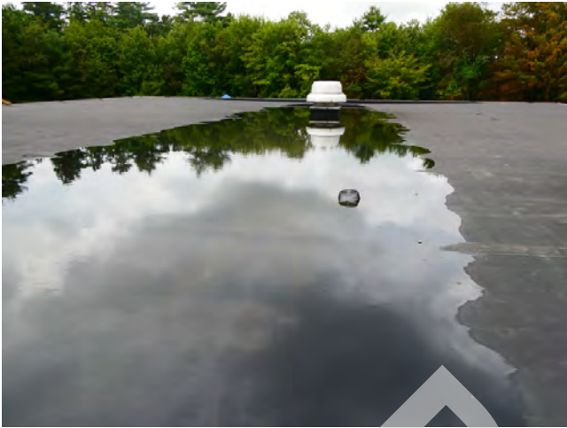
53. Roof - Standing water at northeast roof surface
