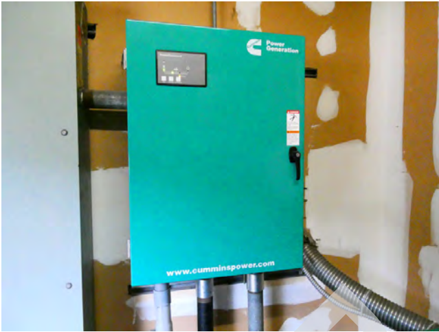
93. MEP - Emergency generator transfer switch
