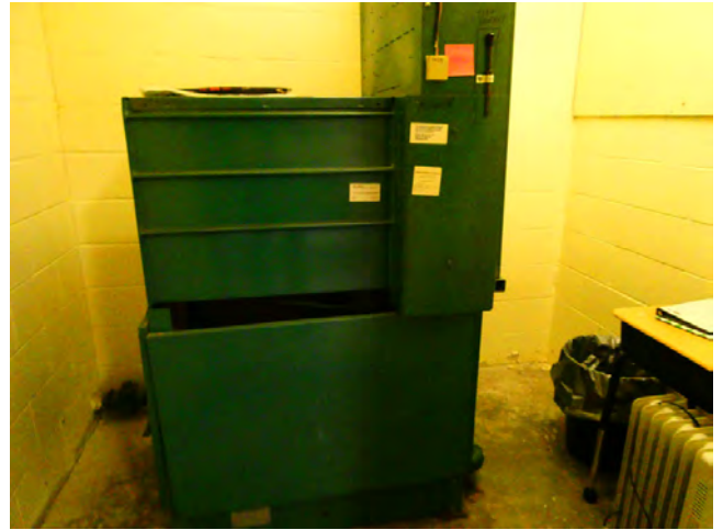
98. Vertical Transportation - Hydraulic elevator equipment
