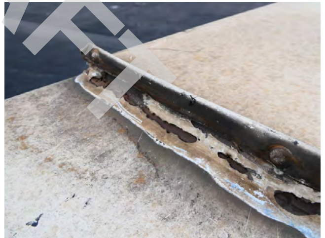
56. Roof - Deteriorated sealants at parapet wall flashing (central roof)
