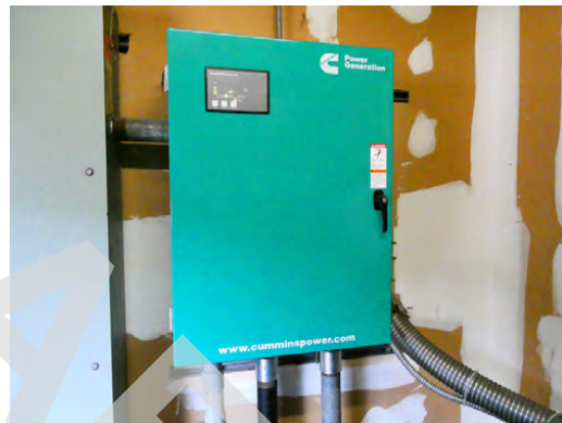
MEP - Emergency generator transfer switch
