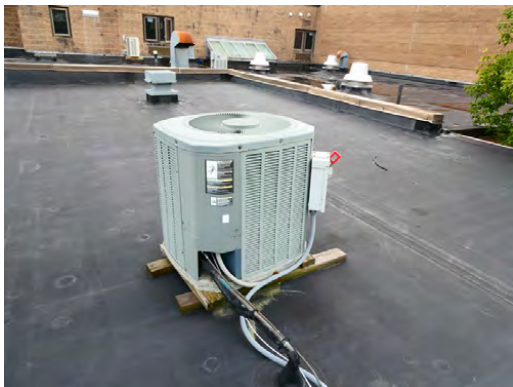
MEP - Roof mounted condensing unit
