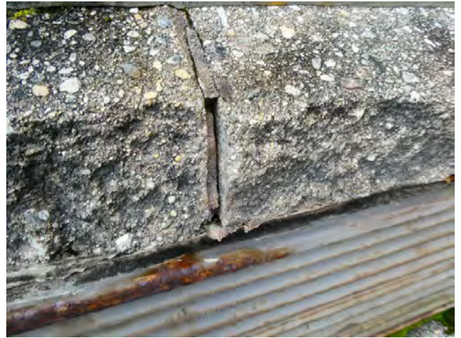
34. Exterior - Deteriorated mortar joints at CMU along roofline
