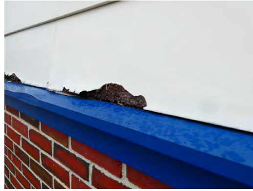
Exterior - Isolated deteriorated wood fiber siding (west elevation)
