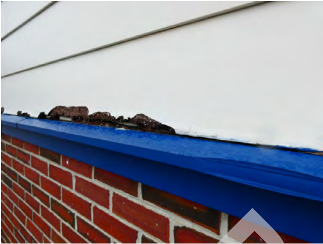
37. Exterior - Isolated deteriorated wood fiber siding (west elevation)
