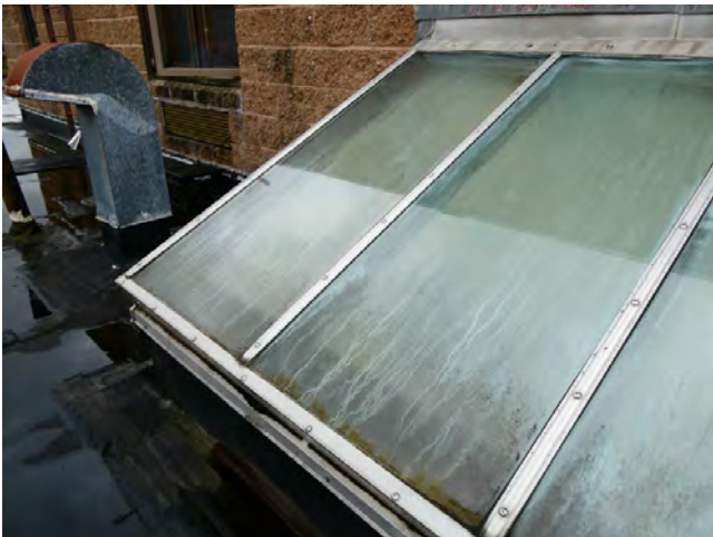
63. Roof - Skylight glazing with fogging condition
