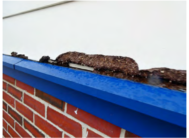
38. Exterior - Isolated deteriorated wood fiber siding (west elevation)
