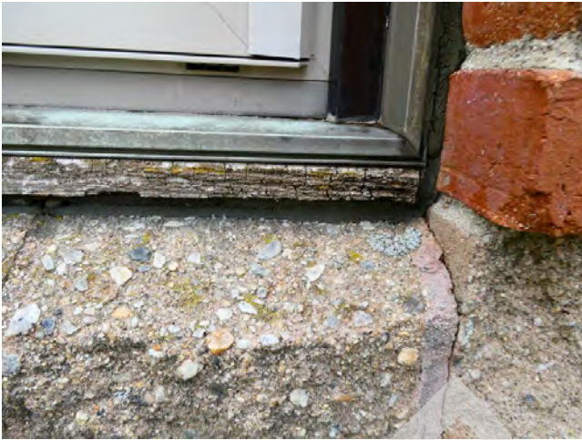
33. Exterior - Deteriorated mortar at southeast elevation
