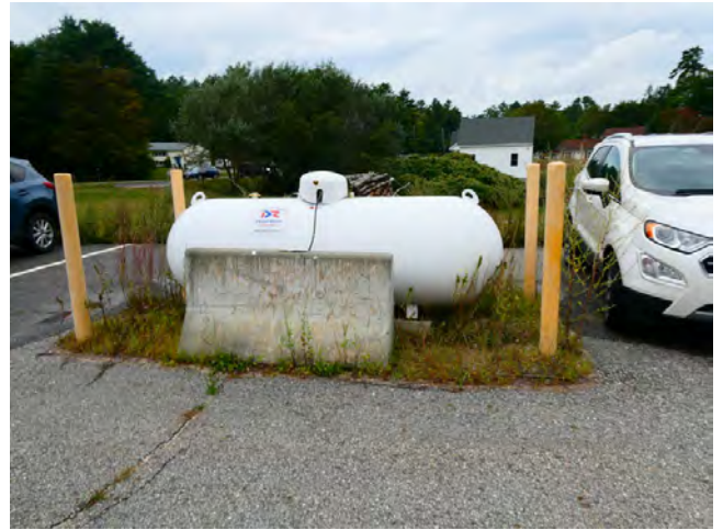
90. MEP - Onsite propane tank
