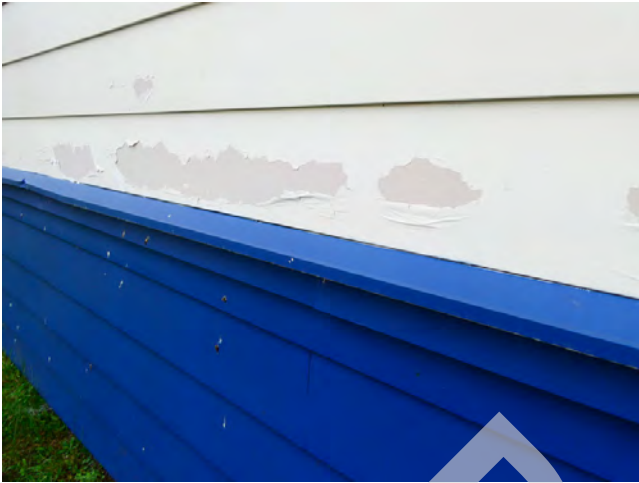
41. Exterior - Worn paint finish along north elevation
