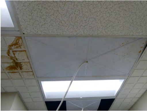
Interiors - Active roof leak at south portion
