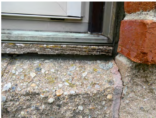
Exterior - Deteriorated mortar at southeast elevation
