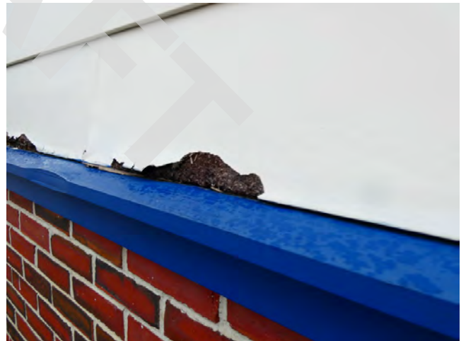
36. Exterior - Isolated deteriorated wood fiber siding (west elevation)
