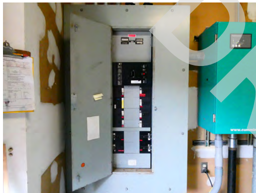
MEP - Main electrical disconnect panel
