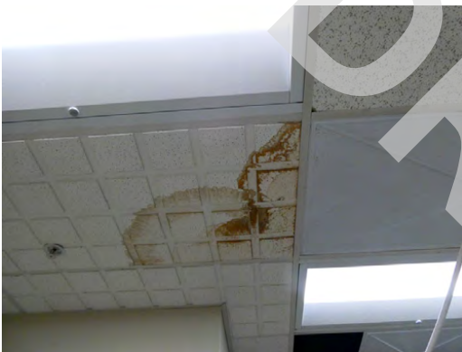
Interiors - Moisture stained ceiling tiles at south portion
