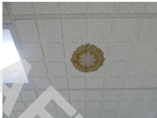
Interiors - Moisture stained ceiling tiles at south portion
