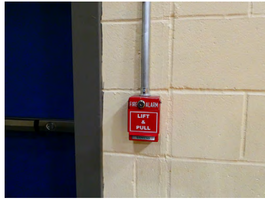
FLS - Fire pull stations located throughout
