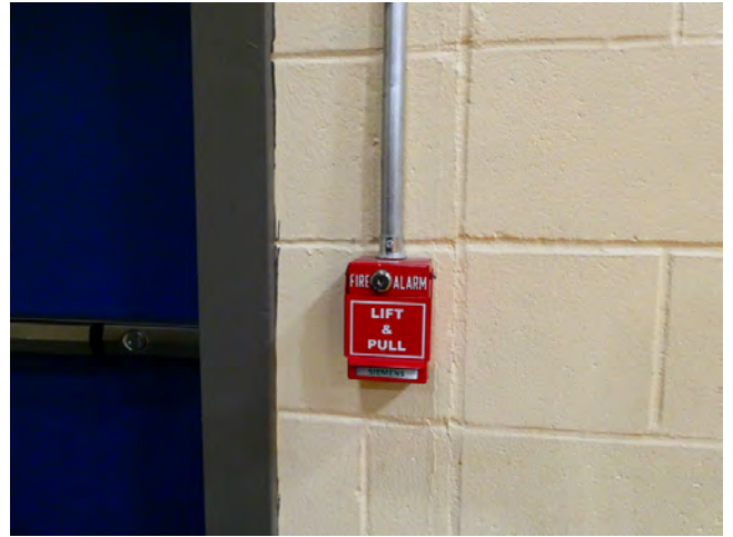
102. FLS - Fire pull stations located throughout
