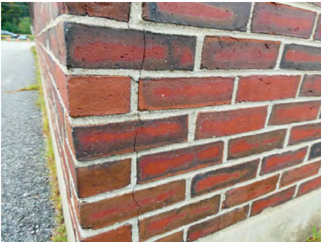
23. Structure - Vertical cracking along brick facade (northeast corner)
