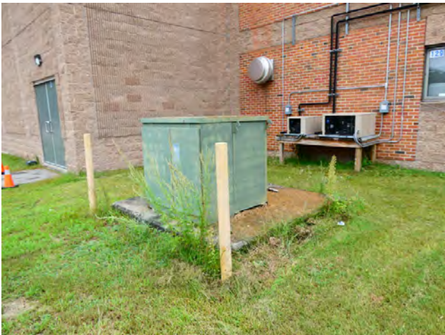
91. MEP - Pad mounted electrical transformer
