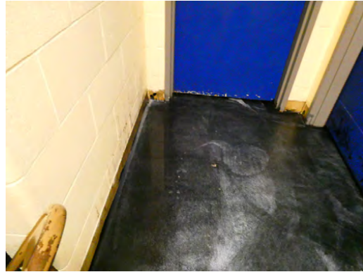
Interiors - Isolated leak at the kitchen bathroom area
