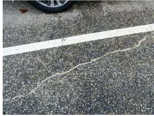
Site - Longitudinal cracking along south parking area
