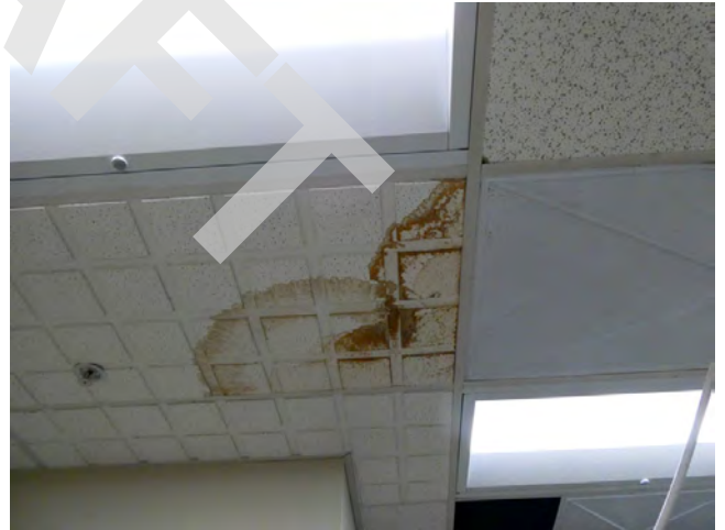
120. Interiors - Moisture stained ceiling tiles at south portion
