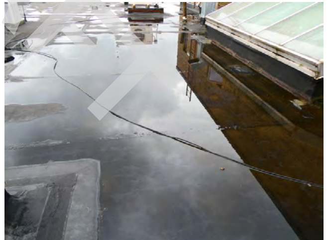
52. Roof - Standing water at central roof surface
