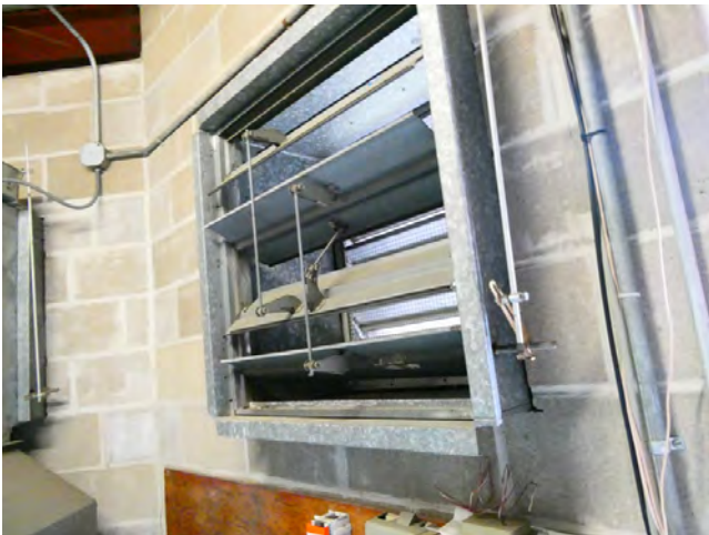
87. MEP - Natural ventilation exhaust in generator room
