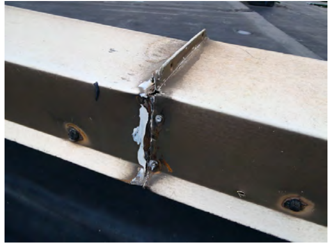
58. Roof - Deteriorated sealants at parapet wall flashing (central roof)
