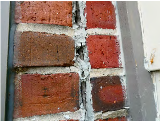
35. Exterior - Deteriorated vertical sealants along north elevation
