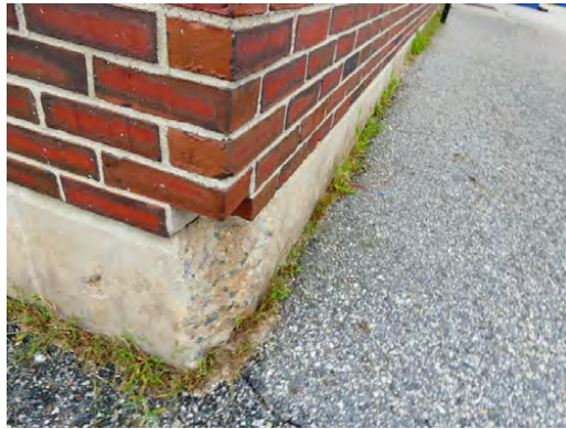
Structure - Damaged section of exposed concrete slab and missing brick
