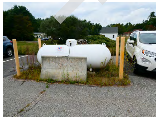
MEP - Onsite propane tank
