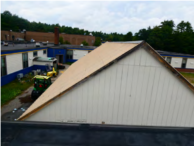
43. Exterior - Deteriorated siding and worn paint at maintenance structure
