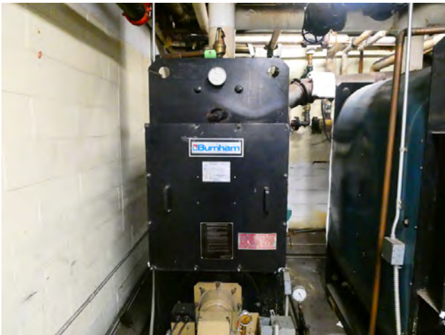
79. MEP - One of two low pressure boilers for heating
