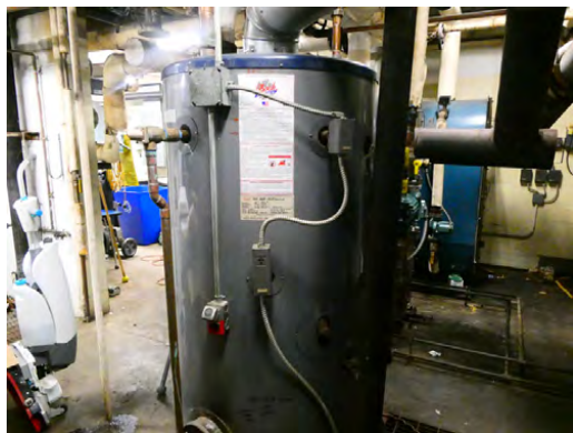
MEP - Gas fired domestic water heater
