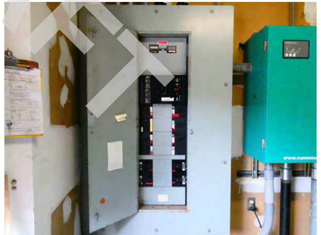
92. MEP - Main electrical disconnect panel
