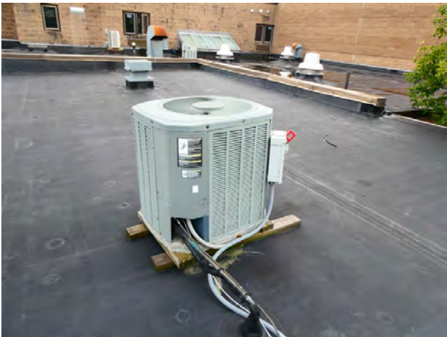
83. MEP - Roof mounted condensing unit
