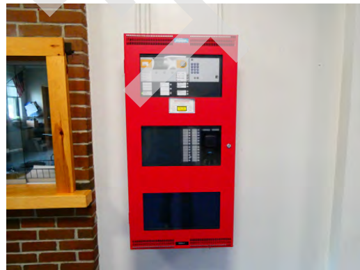
FLS - Main fire alarm control panel
