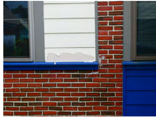
Exterior - Worn paint finish along north elevation
