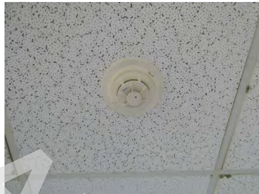
FLS - Hardwired ceiling mounted smoke detectors
