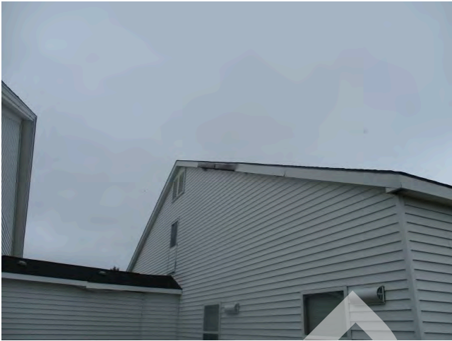
9. Damaged fascia on north end of 1996 addition
