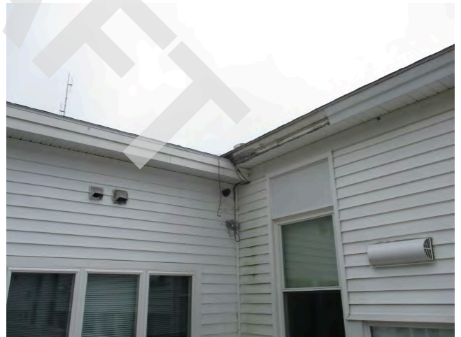
4. Damaged soffit at "problem" leak area near principal's office
