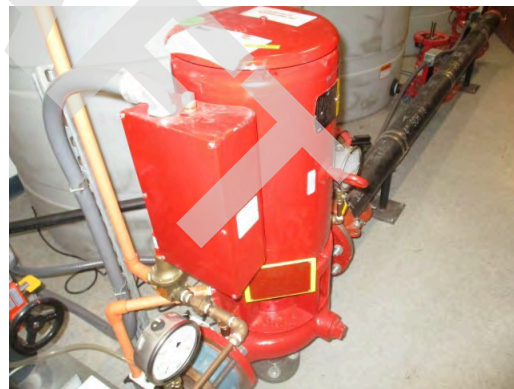
Fire pump in sprinkler room
