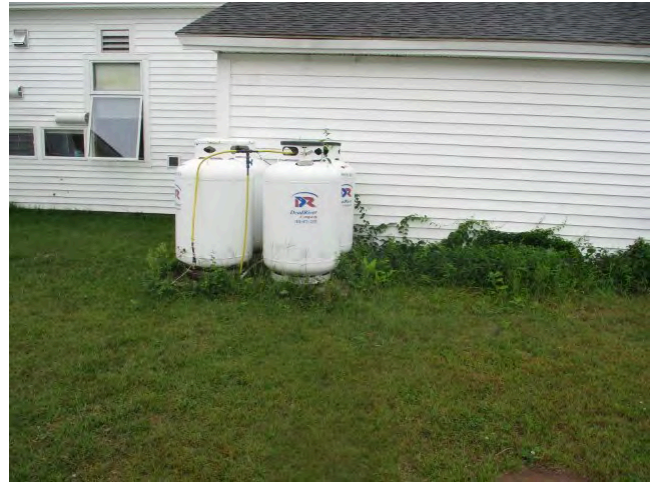
54. Propane tanks south of kitchen
