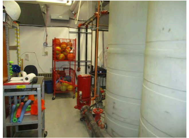
66. Sprinkler room and coach's office
