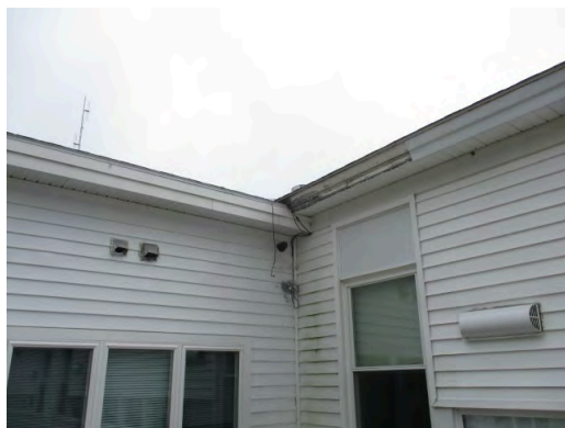
Damaged soffit at "problem" leak area near principal's office
