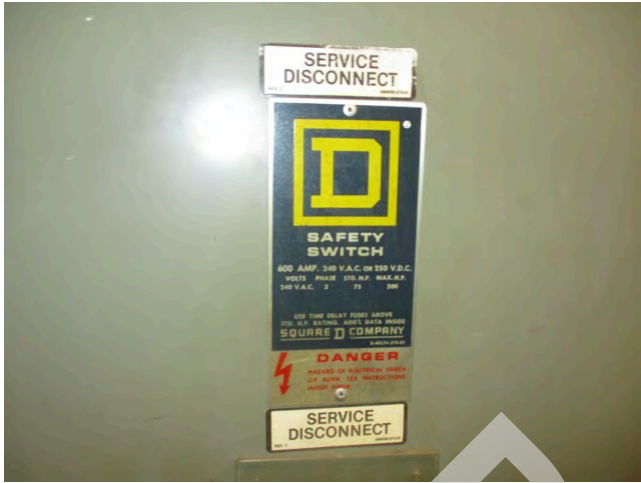
61. Main electrical disconnect
