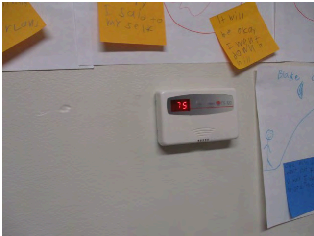
47. Thermostat in classroom 228
