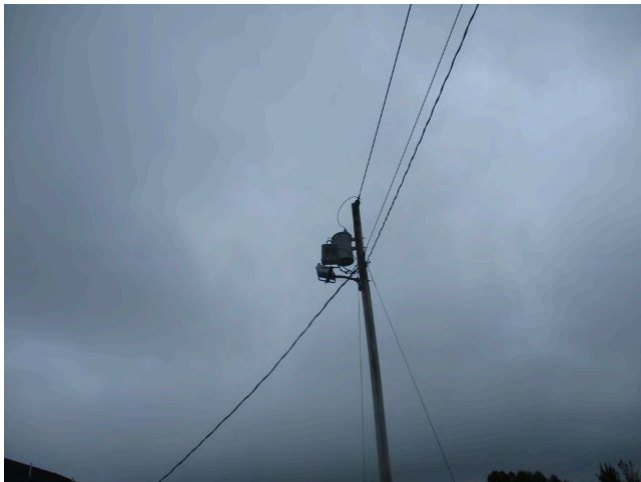
63. Pole-mounted transformer west of building
