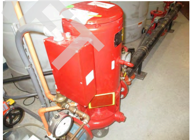
68. Fire pump in sprinkler room
