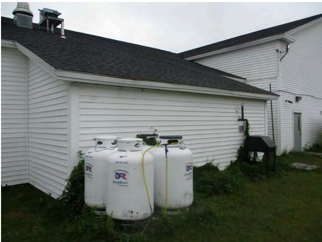
43. Oil tank enclosure south of boiler room
