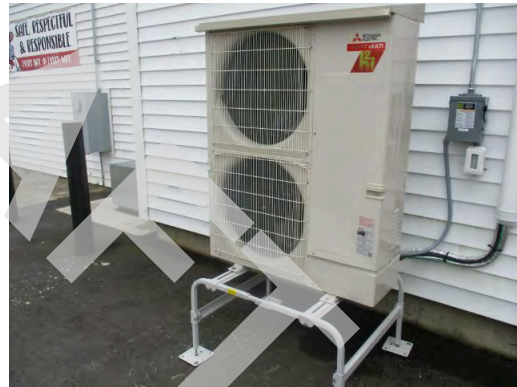
Split system condenser near main entrance
