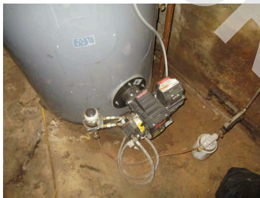
Oil-fired water heater in boiler room
