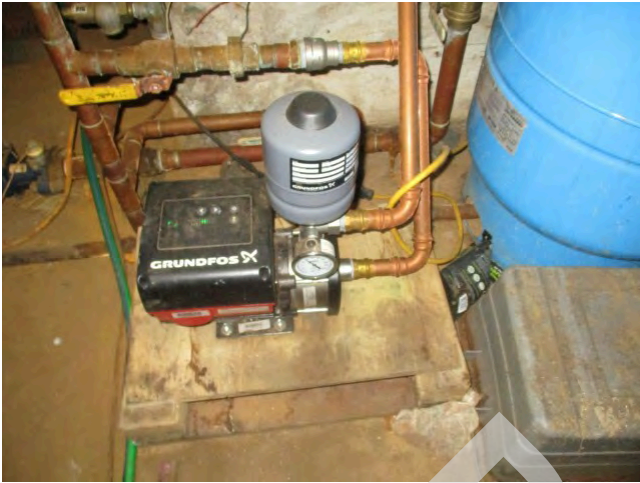
57. Domestic water pump in boiler room
