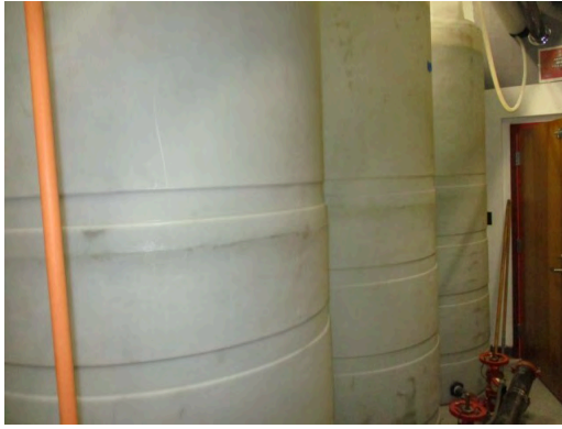
Fire sprinkler water storage tanks
