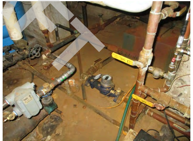
56. Domestic water meter in boiler room
