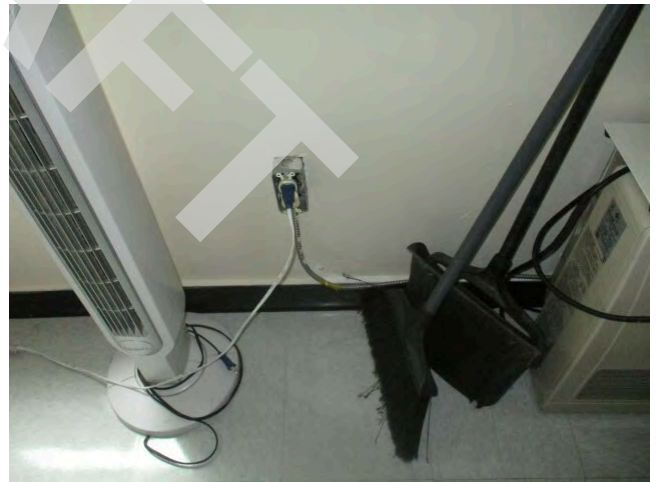
64. Classroom 226 exposed outlet
