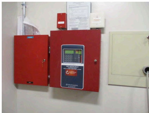
Fire alarm panel in main office
