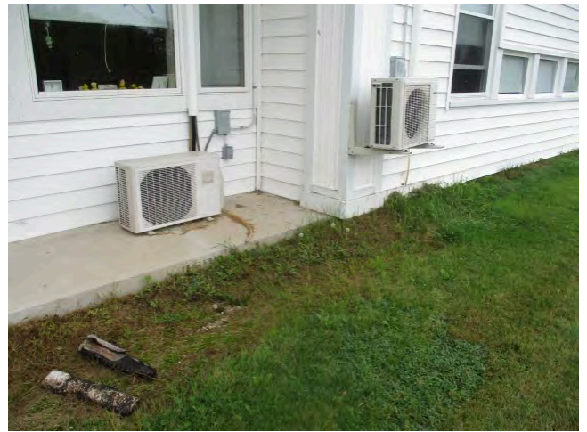
46. Split system condensing units on west side of building
