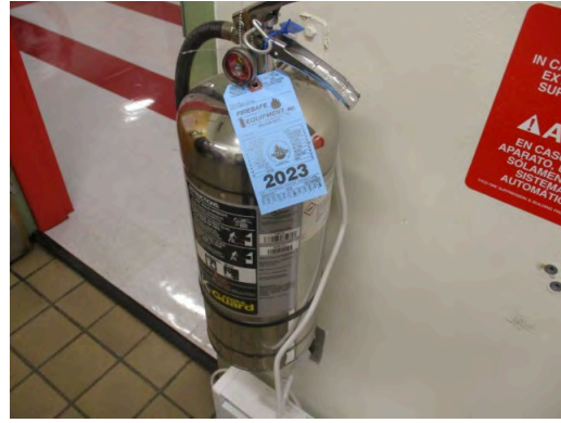
Typical fire extinguisher
