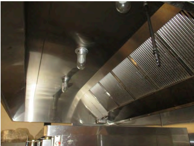
71. Ansul system in kitchen hood
