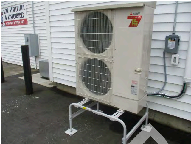
45. Split system condenser near main entrance
