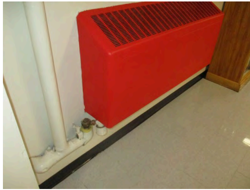
Typical slant-front radiator
