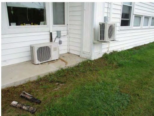
Split system condensing units on west side of building
