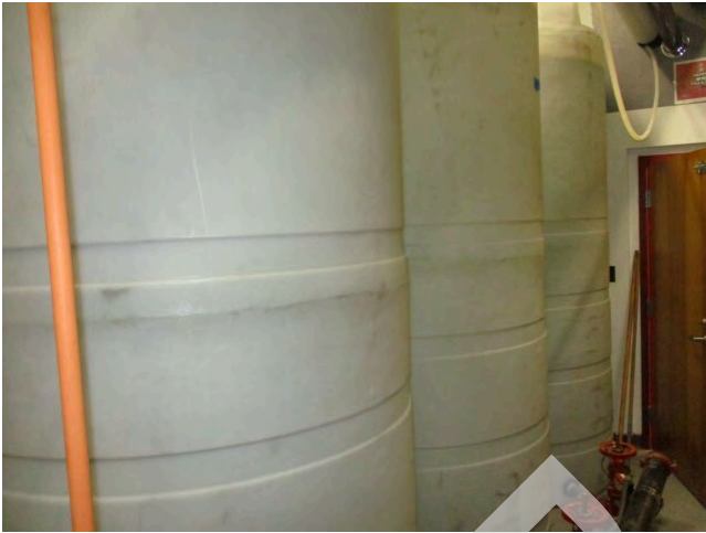
69. Fire sprinkler water storage tanks
