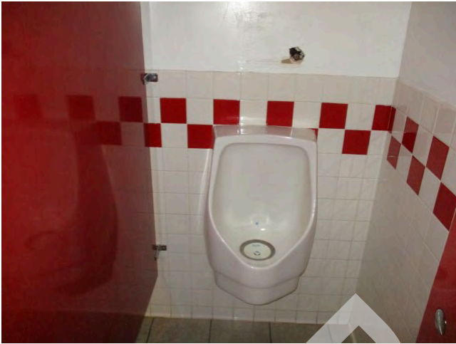
77. Waterless urinal in boy's restroom near main office
