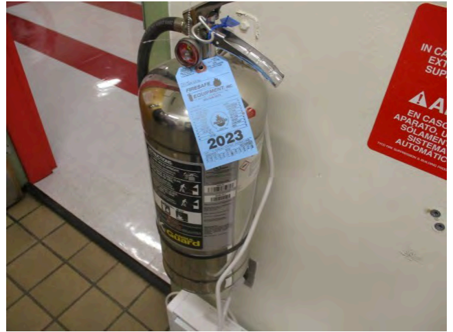
70. Typical fire extinguisher
