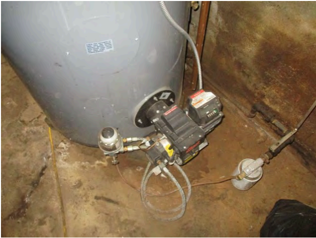
58. Oil-fired water heater in boiler room
