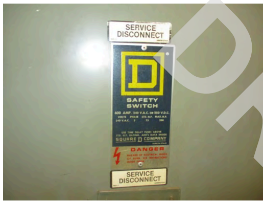
Main electrical disconnect
