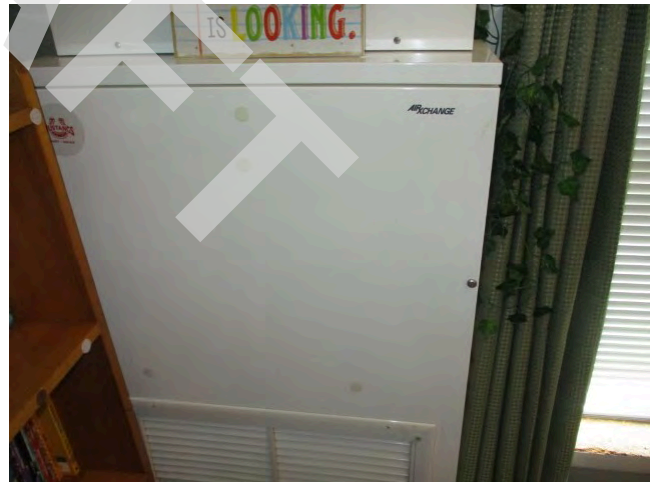
52. Air exchange unit in classroom 230
