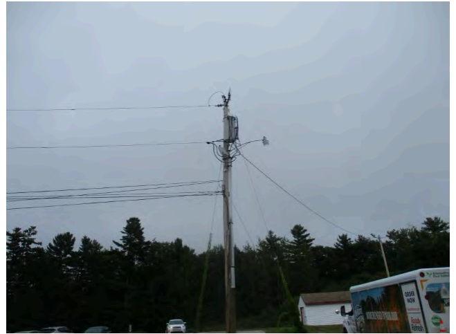
62. Pole-mount transformer in parking area
