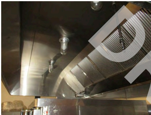
Ansul system in kitchen hood
