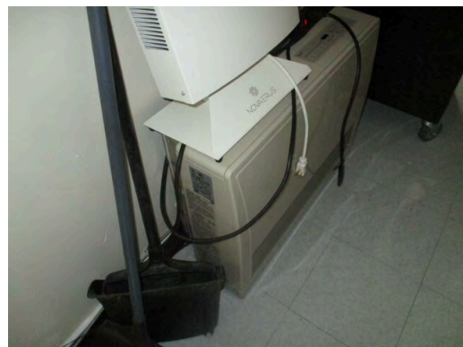
Typical Rinnai heater in classroom 226
