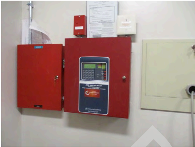
65. Fire alarm panel in main office
