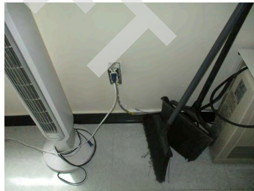
Classroom 226 exposed outlet
