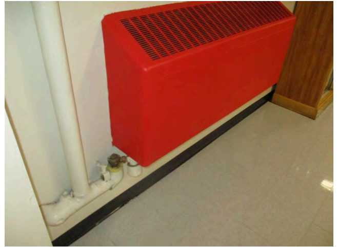
50. Typical slant-front radiator
