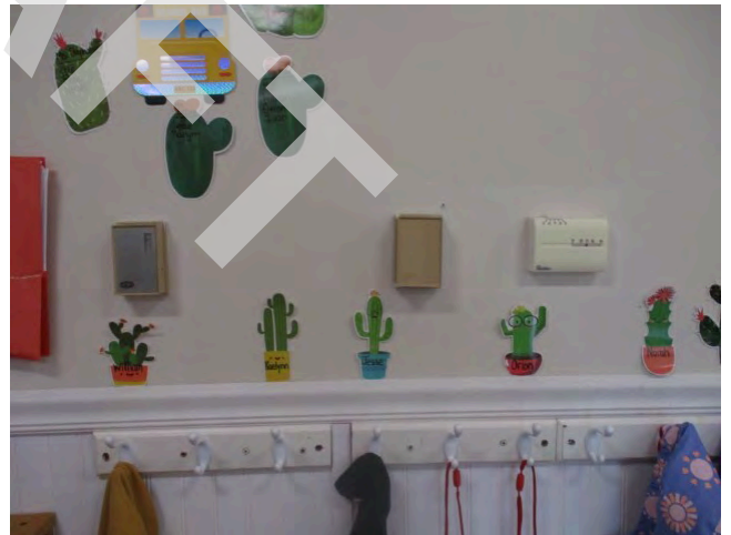
48. Thermostats in classroom 223
