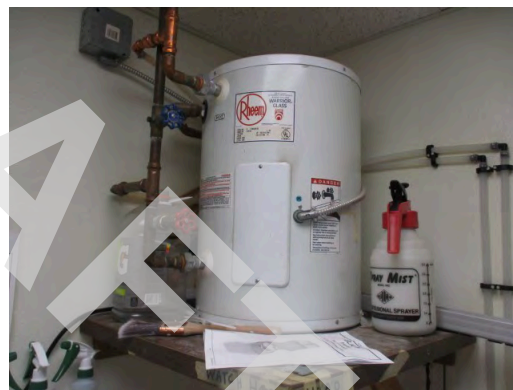
Water heater in 1996 addition
