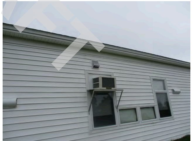
44. Window AC on west side of building
