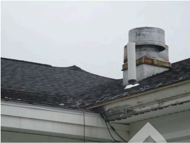
41. Roofing and heat tape at "problem" area near principal's office
