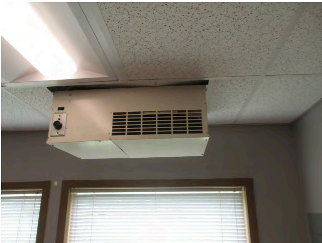
51. Ventilator in room 227
