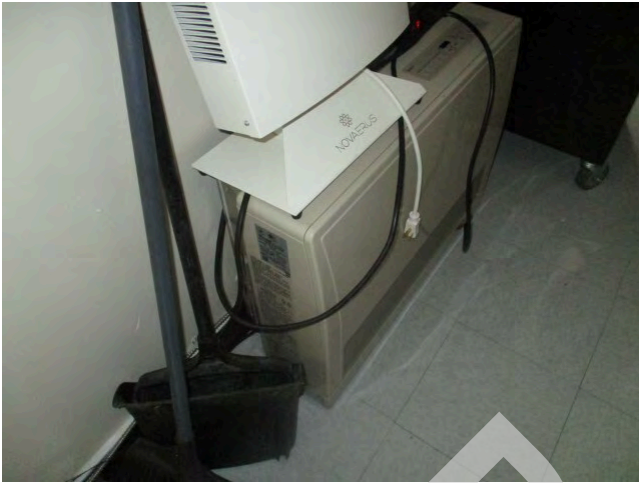
49. Typical Rinnai heater in classroom 226
