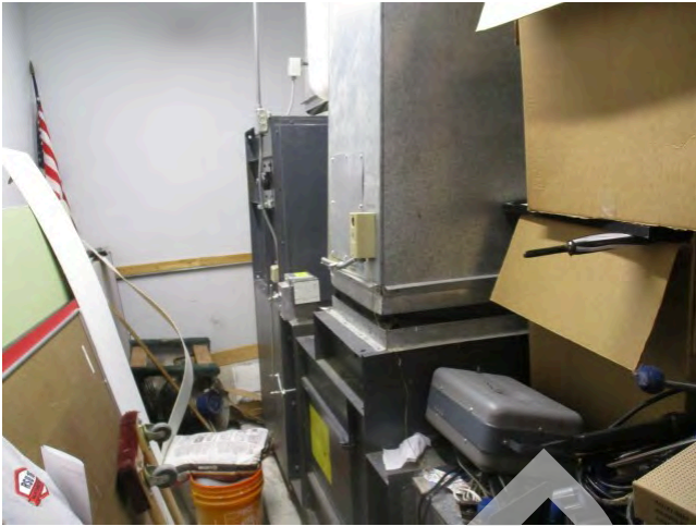
53. Economizer air handler near gymnasium
