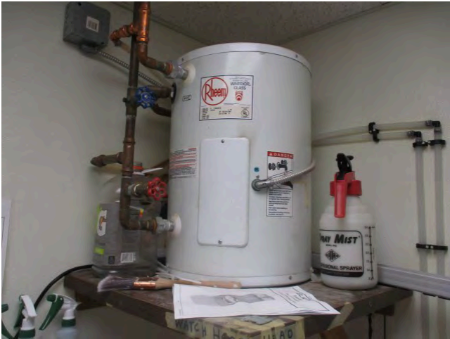
59. Water heater in 1996 addition
