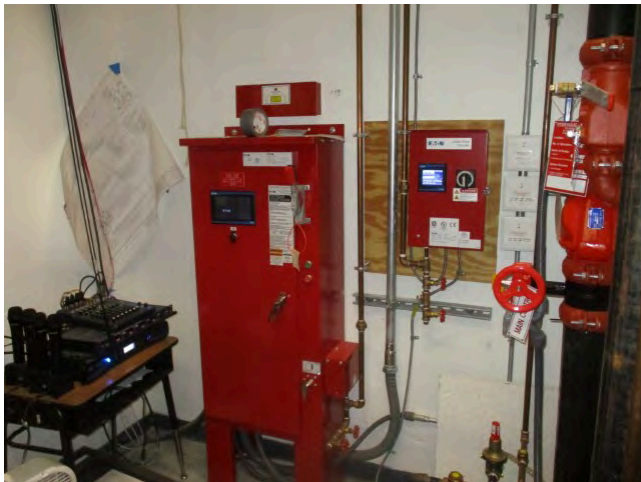
67. Fire pump controller
