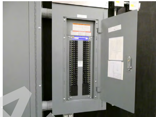
MEP - Typical electrical breaker panel
