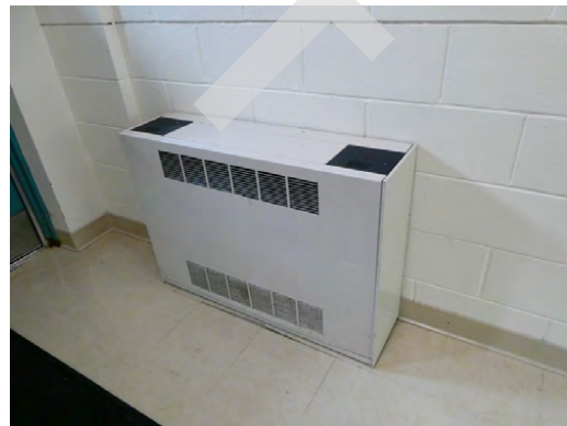
MEP - Wall mounted cabinet forced air units
