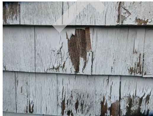
Exterior - Deteriorated stain finish at wood siding
