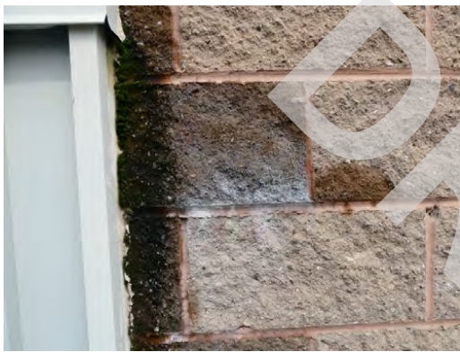
Exterior - Moisture staining at east elevation (roofline)
