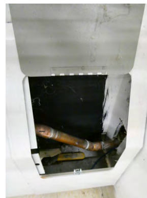
MEP - Copper piping for hydronic system
