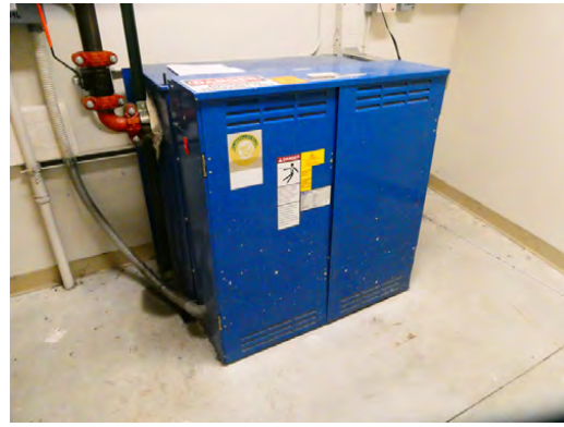
Vertical Transportation - Hydraulic elevator equipment
