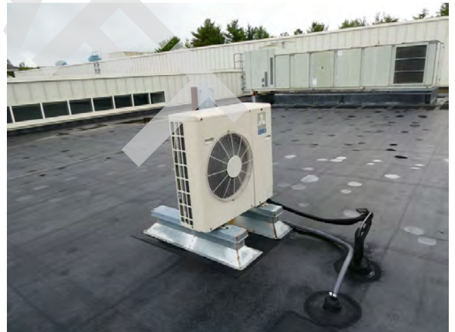
120. MEP - Older roof mounted heat pump for ductless system
