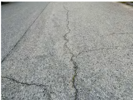
Site - Longitudinal cracking along asphalt pavement
