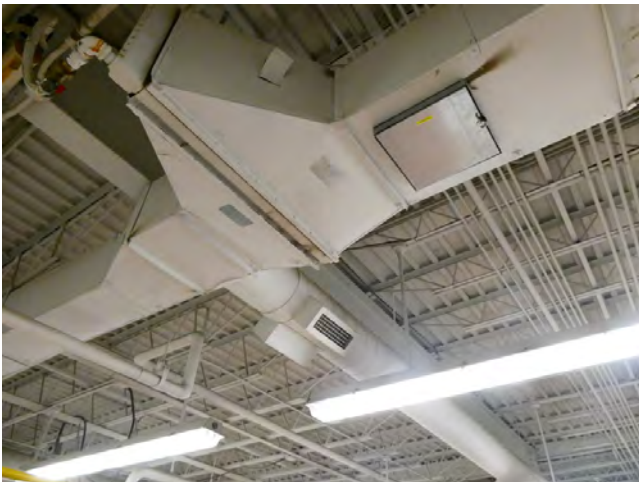
131. MEP - Middle school gymnasium ducting system
