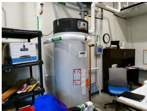
MEP - Propane sourced domestic water heater for middle school
