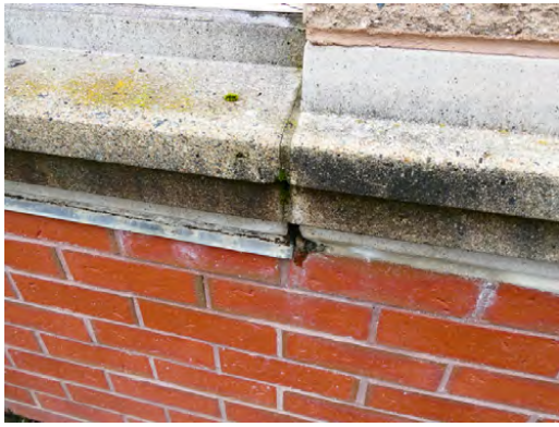
Exterior - Moisture staining along concrete window sill (courtyard)
