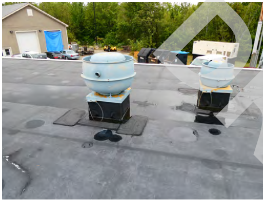
MEP - Upblast roof exhaust fans for the kitchen
