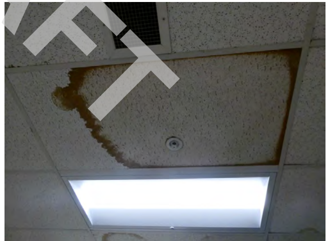
156. Interiors - Moisture damaged ceiling panel from prior leak
