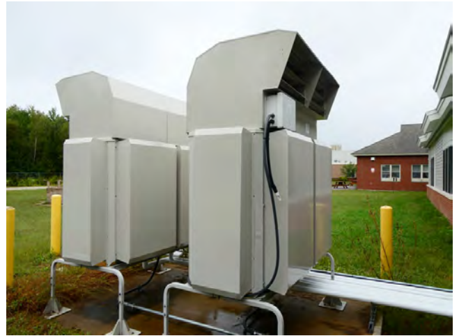
126. MEP - VRF heat pumps for the middle school
