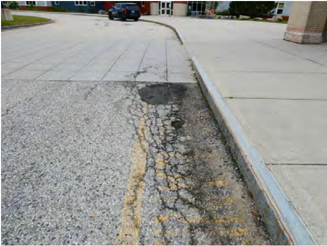
10. Site - Area of asphalt deterioration at main drive
