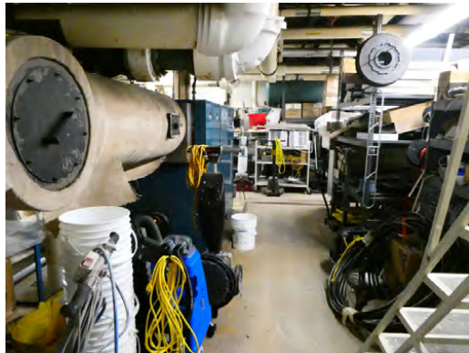
Interiors - Main boiler room and equipment
