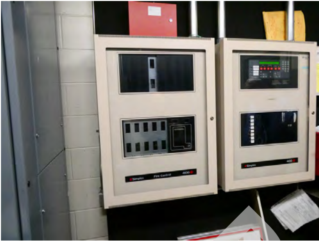
149. FLS - Main fire alarm control panels
