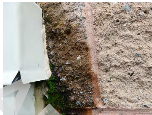
Exterior - Moisture staining at east elevation (roofline)
