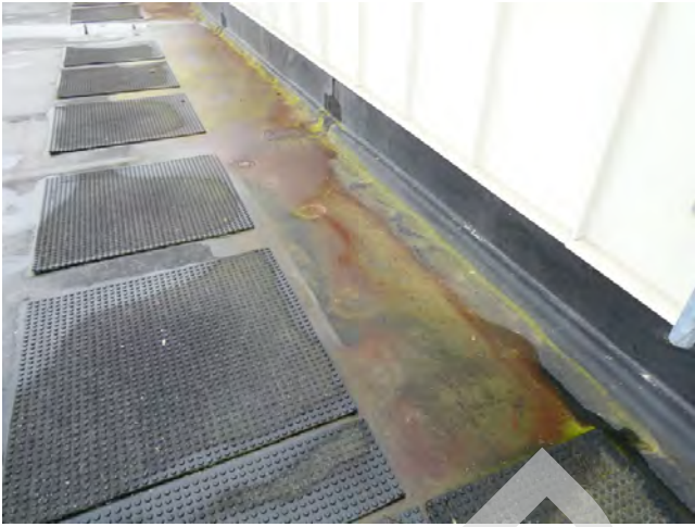
65. Roof - Organic growth along central roof section
