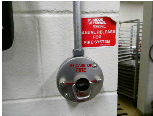
FLS - ANSUL fire suppression pull station
