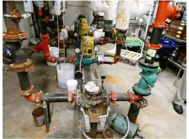
114. MEP - Circulation pumps for the boiler systems
