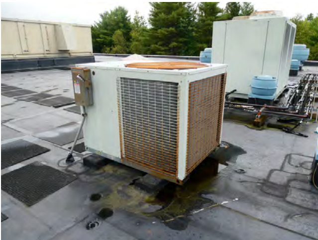
123. MEP - Older roof mounted air cooled condenser
