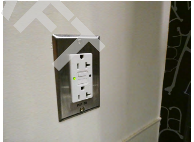
136. MEP - GFCI outlets in wet locations
