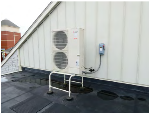
MEP - Newer roof mounted heat pump for ductless system
