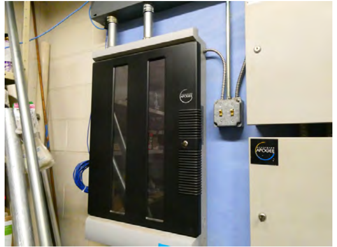
130. MEP - Building management system controls
