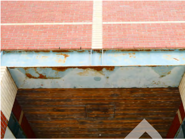
53. Exterior - Surface corrosion along steel framing for covered entryway
