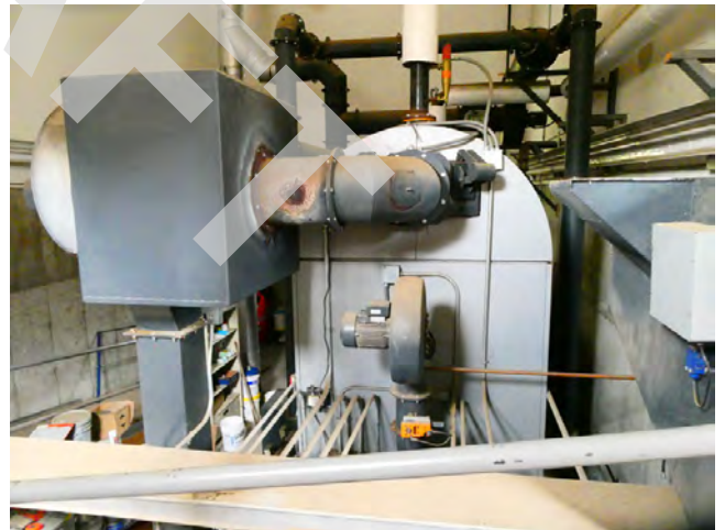
112. MEP - Biomass heating system
