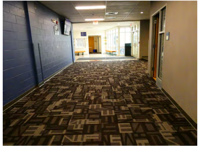
94. Interiors - Isolated areas of commercial carpeting in common areas
