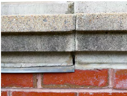
Exterior - Deteriorated mortar joints at courtyard exterior
