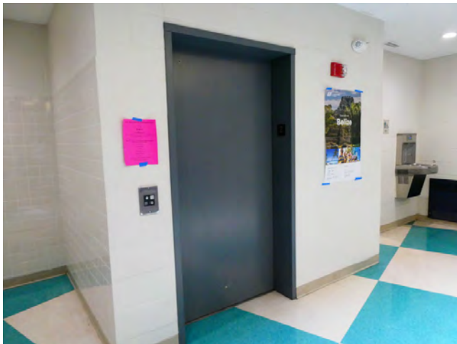
139. Vertical Transportation - Elevator for the high school area
