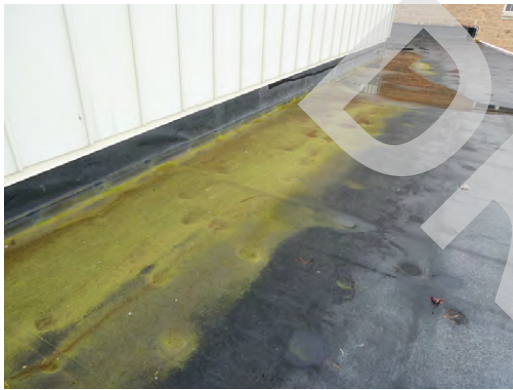
Roof - Organic growth along southwest roof section
