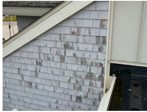
Exterior - Deteriorated stain finish at wood siding
