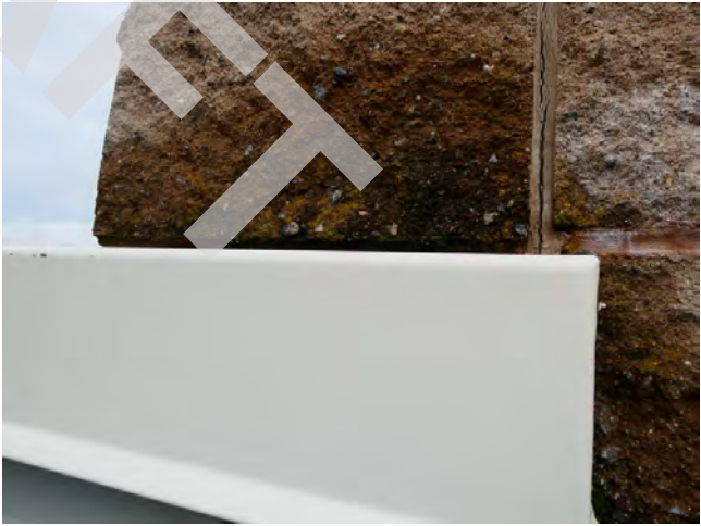
48. Exterior - Moisture staining and deteriorated sealants at east elevation (roofline)
