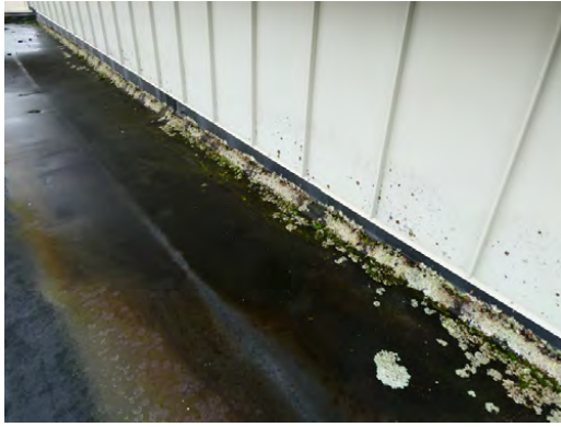
Roof - Organic growth along central roof section
