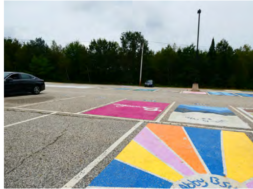
Site - North parking surface condition
