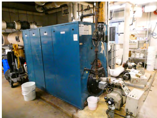
MEP - One of two low pressure boilers for heating
