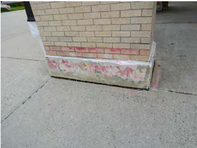
35. Exterior - Deteriorated EIFS at base of columns (main entrance)
