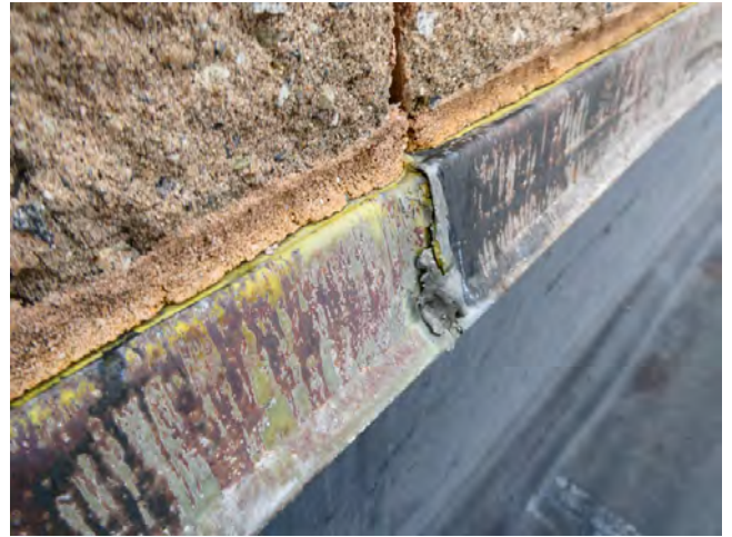
58. Roof - Deteriorated sealants at parapet flashing (south portion)
