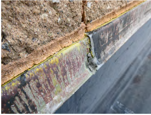
Roof - Deteriorated sealants at parapet flashing (south portion)
