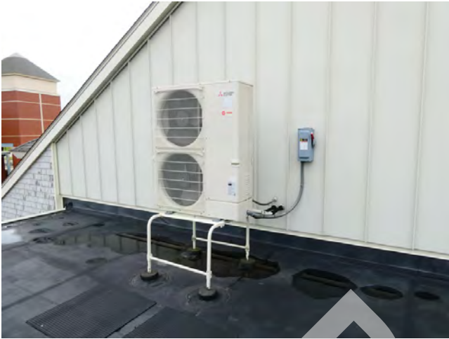
121. MEP - Newer roof mounted heat pump for ductless system
