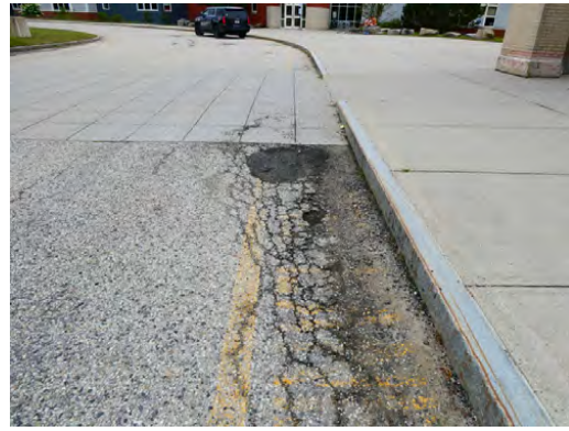
Site - Area of asphalt deterioration at main drive
