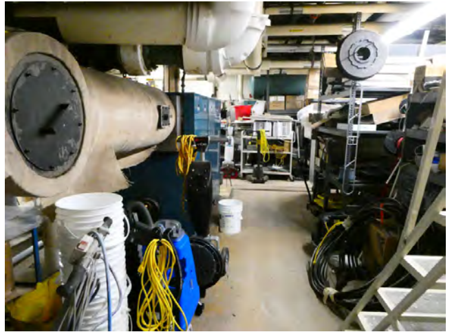
150. Interiors - Main boiler room and equipment
