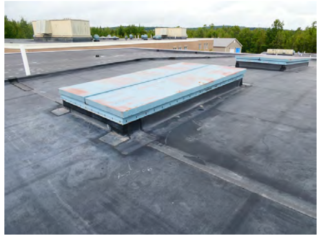
74. Roof - Smoke exhaust system for auditorium
