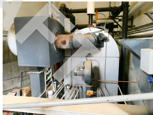
MEP - Biomass heating system
