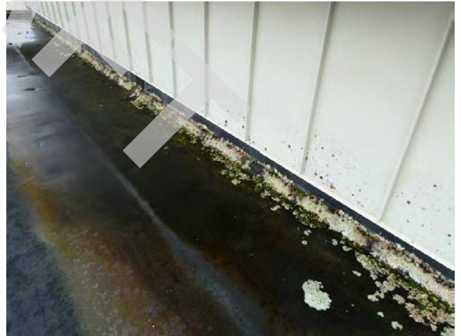
64. Roof - Organic growth along central roof section
