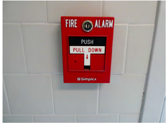
146. FLS - Fire pull stations in common areas
