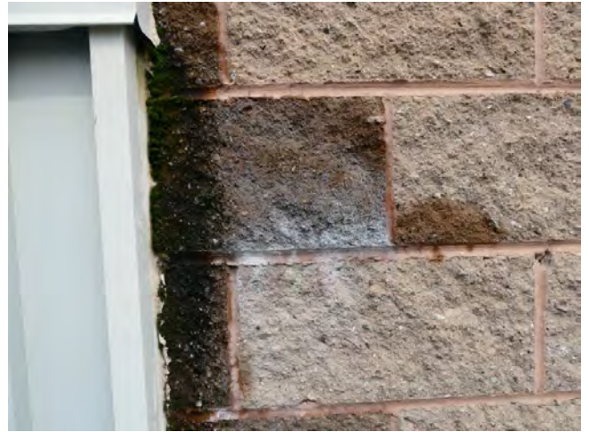
50. Exterior - Moisture staining at east elevation (roofline)
