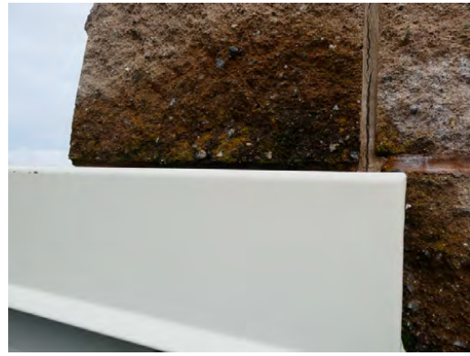
Exterior - Moisture staining and deteriorated sealants at east elevation (roofline)
