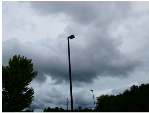
Site - Pole mounted lighting fixtures for parking area
