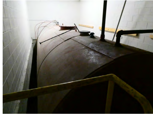
MEP - Interior oil storage tank
