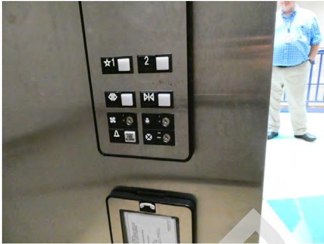
137. Vertical Transportation - Elevator controls
