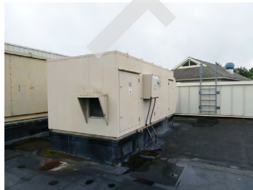
MEP - Roof mounted air recovery unit
