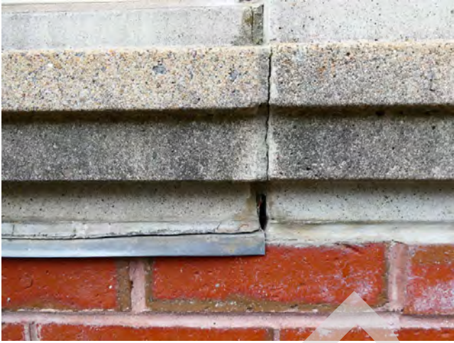
37. Exterior - Deteriorated mortar joints at courtyard exterior
