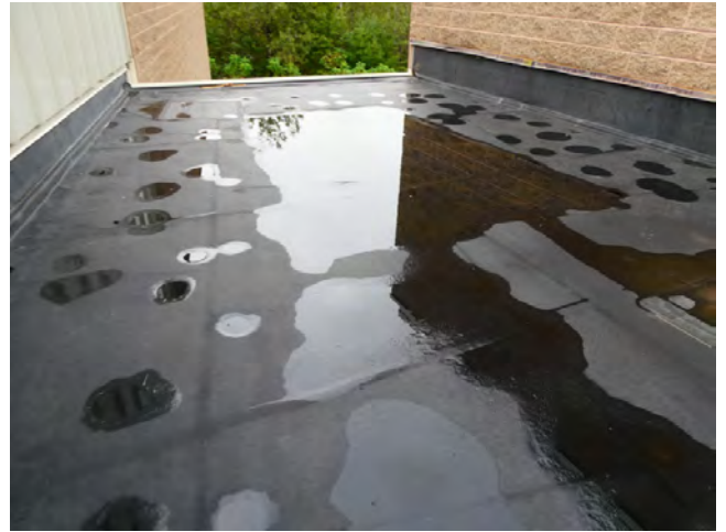
62. Roof - Isolated ponding water along southwest roof section
