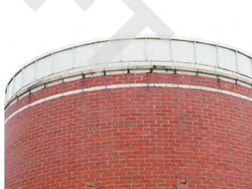
Exterior - Moisture staining along concrete details at middle school entry
