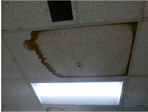
Interiors - Moisture damaged ceiling panel from prior leak
