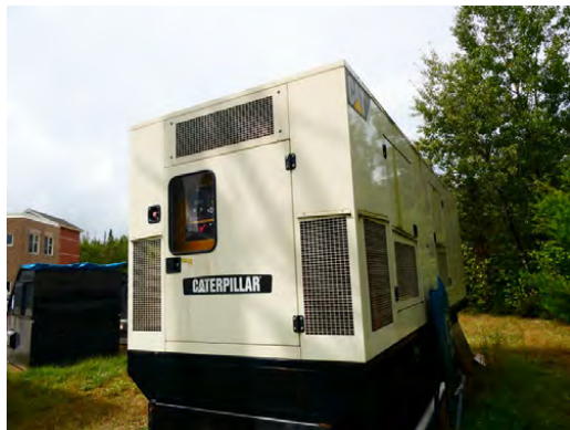
MEP - Emergency electrical generator
