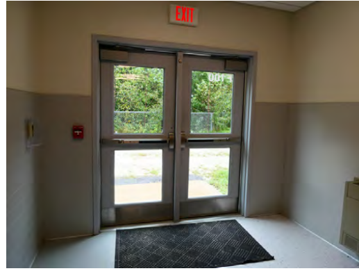
FLS - Lighted emergency exit signage
