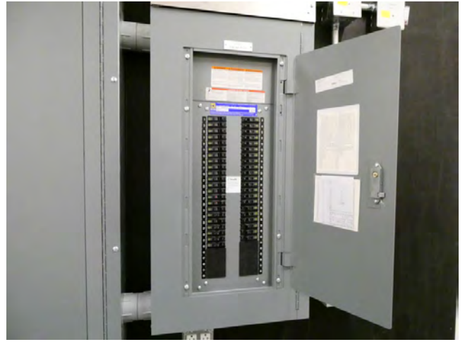
134. MEP - Typical electrical breaker panel
