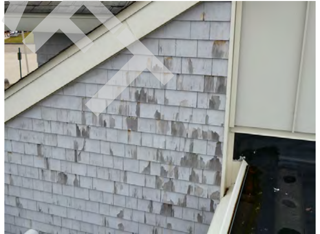
40. Exterior - Deteriorated stain finish at wood siding
