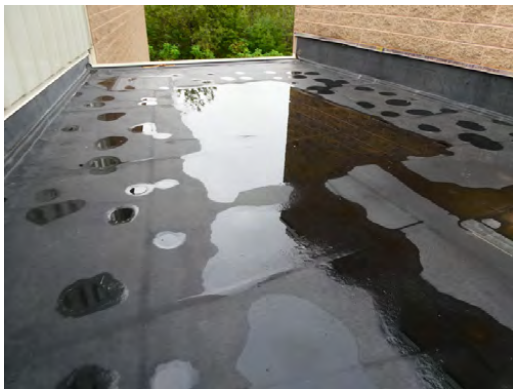
Roof - Isolated ponding water along southwest roof section
