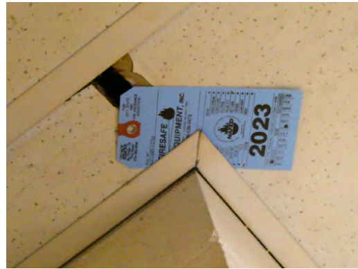
FLS - ANSUL fire suppression system concealed in ceiling
