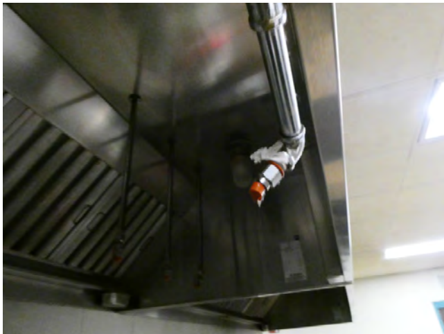
143. FLS - ANSUL suppression system at kitchen hood
