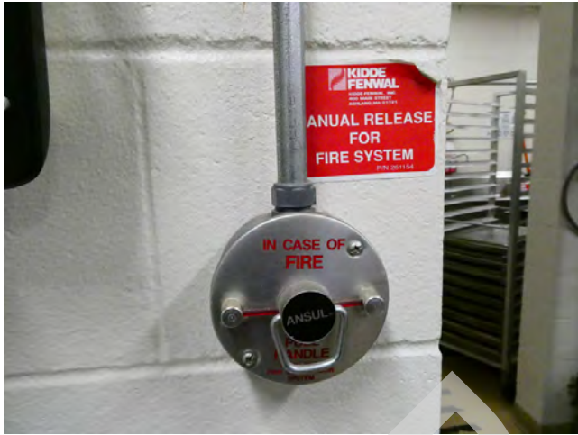
141. FLS - ANSUL fire suppression pull station
