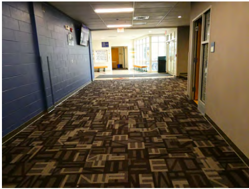
Interiors - Isolated areas of commercial carpeting in common areas
