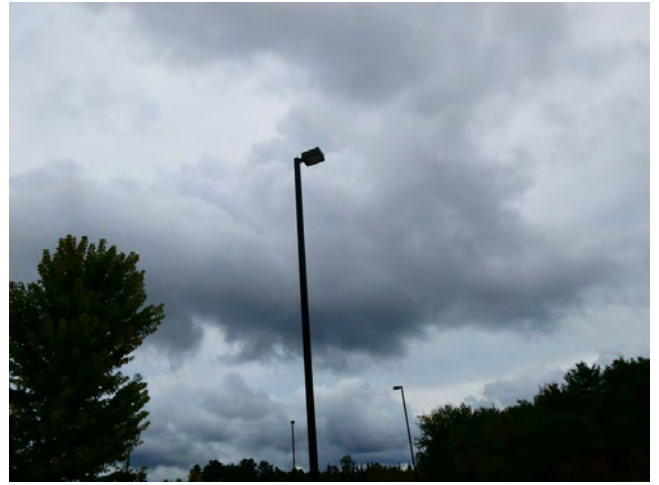
14. Site - Pole mounted lighting fixtures for parking area
