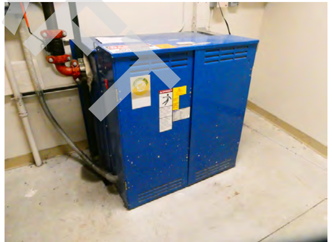
140. Vertical Transportation - Hydraulic elevator equipment
