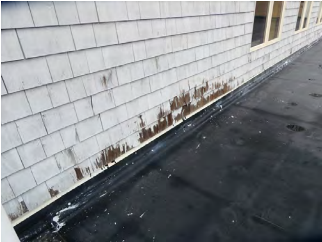
39. Exterior - Deteriorated stain finish at wood siding
