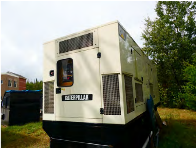
135. MEP - Emergency electrical generator
