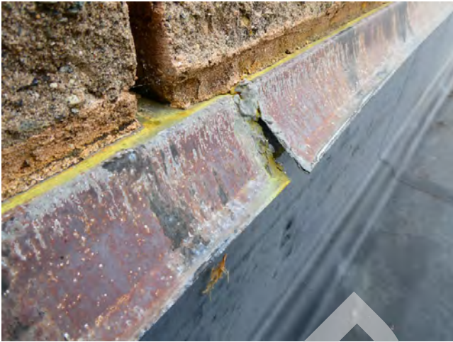
57. Roof - Deteriorated sealants at parapet flashing (south portion)
