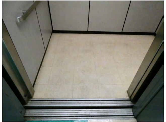
138. Vertical Transportation - Elevator finishes
