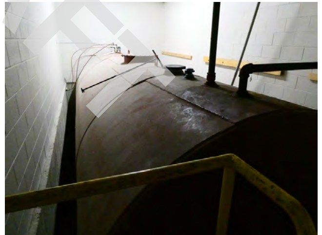
108. MEP - Interior oil storage tank
