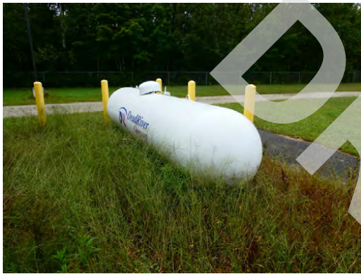
MEP - Onsite propane tank for fuel
