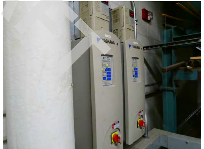
116. MEP - Hot water pump drive systems
