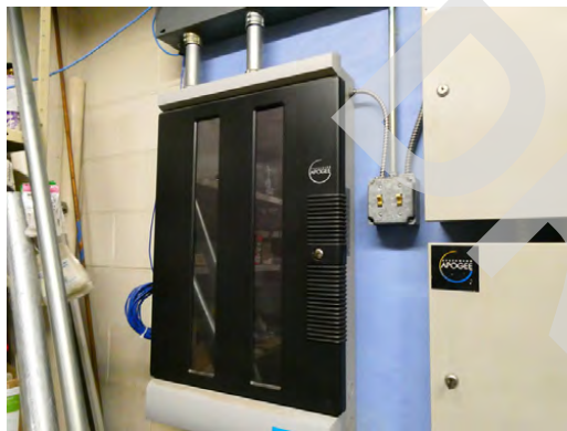
MEP - Building management system controls
