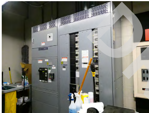
MEP - Main electrical switchboard
