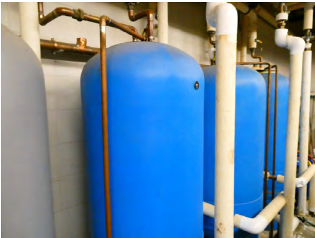
107. MEP - One of three indirect fired water heaters
