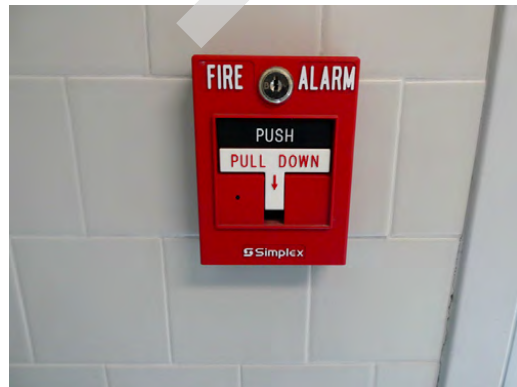
FLS - Fire pull stations in common areas
