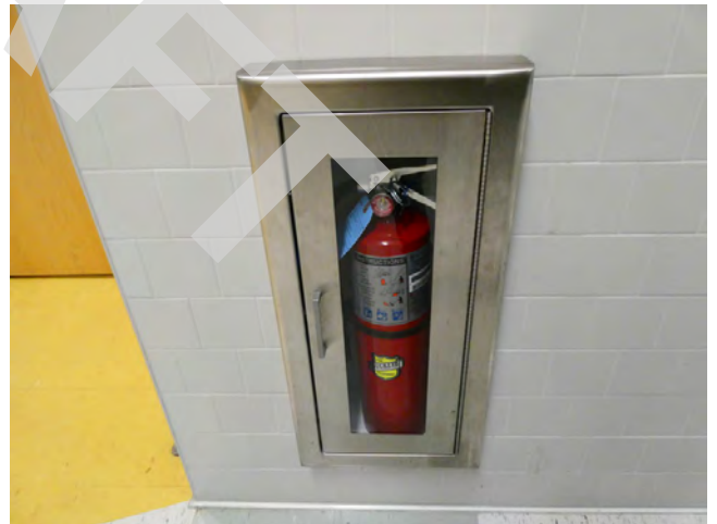
144. FLS - Cabinet mounted fire extinguishers in common areas
