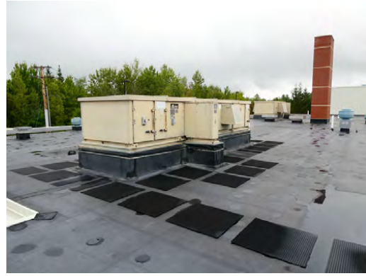
MEP - Packaged roof top unit
