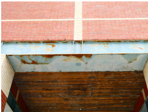
Exterior - Surface corrosion along steel framing for covered entryway
