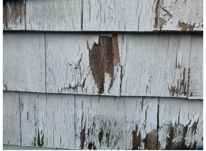
38. Exterior - Deteriorated stain finish at wood siding
