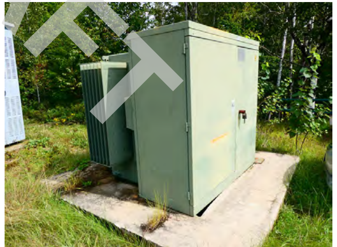
132. MEP - Pad mounted electrical transformer
