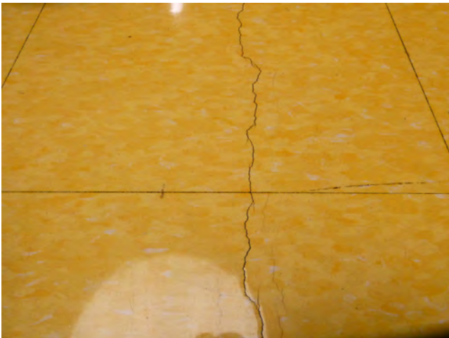
95. Interiors - Isolated areas of stress cracking at common area vinyl flooring
