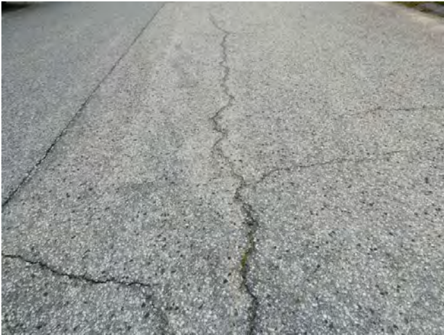
7. Site - Longitudinal cracking along asphalt pavement
