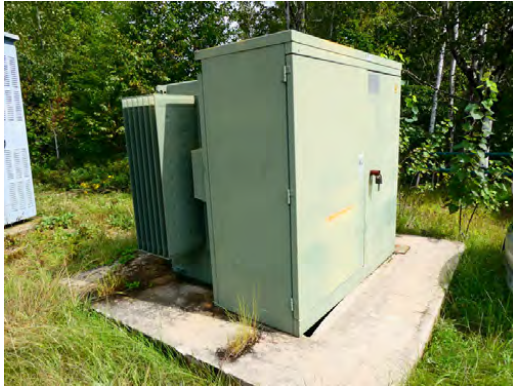
MEP - Pad mounted electrical transformer
