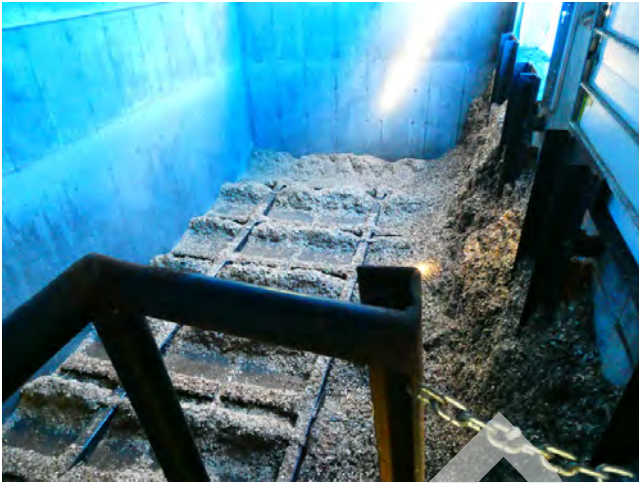
113. MEP - Biomass supply hopper
