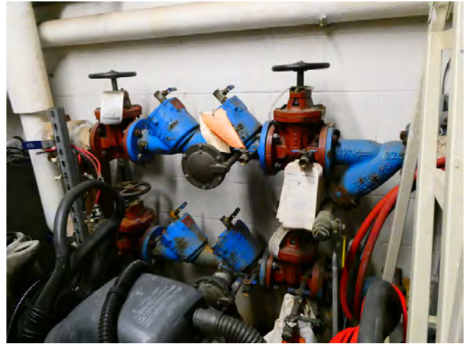
110. MEP - Backflow preventer in mechanical room
