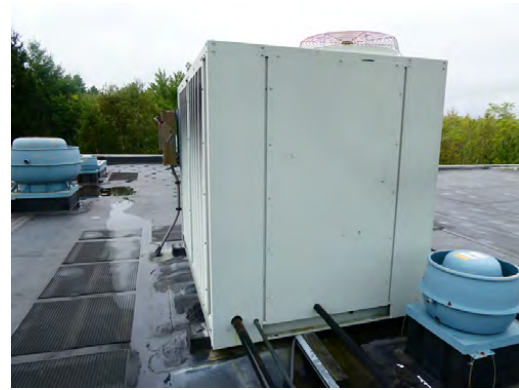
MEP - Roof mounted air cooled packaged chiller
