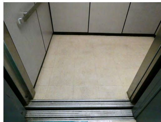
Vertical Transportation - Elevator finishes
