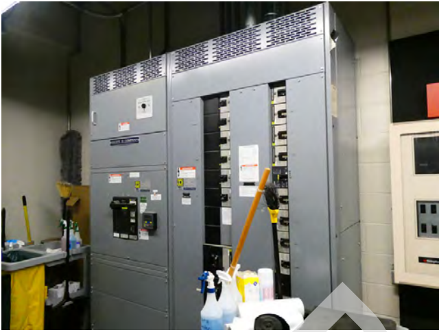
133. MEP - Main electrical switchboard
