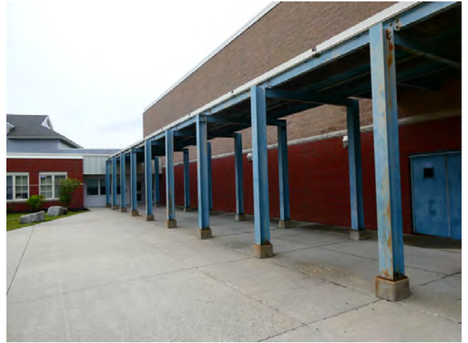
54. Exterior - Surface corrosion along steel framing for covered entryway
