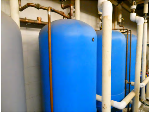
MEP - One of three indirect fired water heaters
