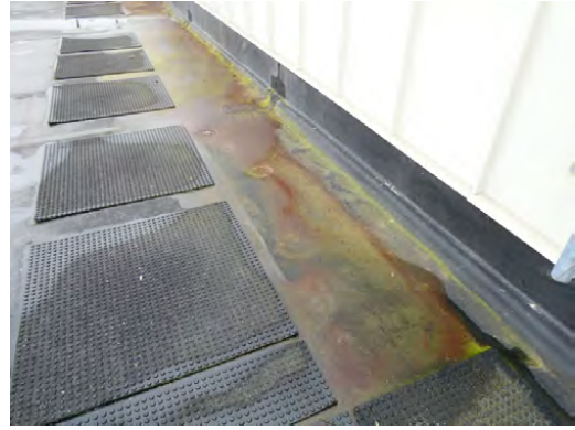
Roof - Organic growth along central roof section
