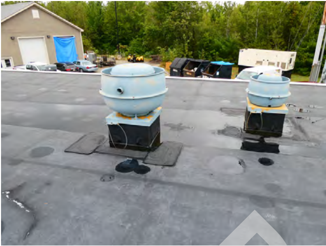
125. MEP - Upblast roof exhaust fans for the kitchen
