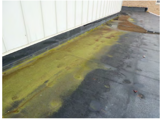
66. Roof - Organic growth along southwest roof section
