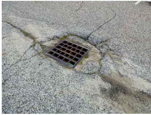
Site - Asphalt pavement condition at north parking area
