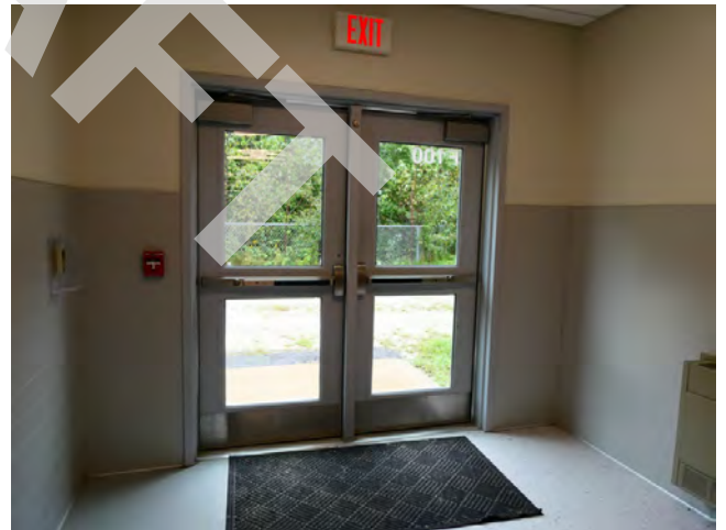
148. FLS - Lighted emergency exit signage
