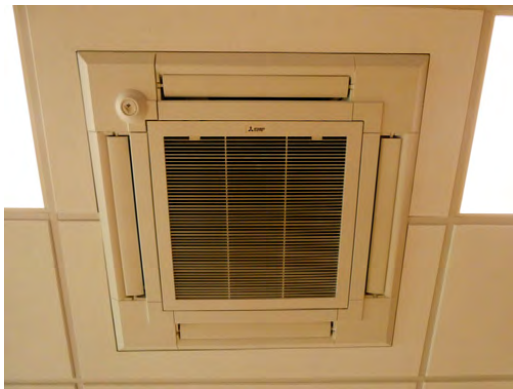
MEP - VRF interior unit type
