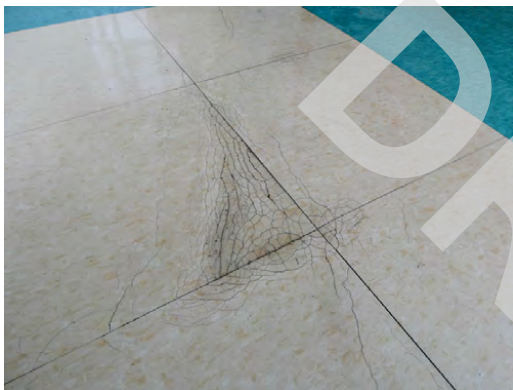
Interiors - Isolated areas of stress cracking at common area vinyl flooring
