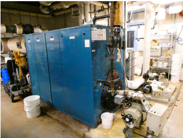
111. MEP - One of two low pressure boilers for heating
