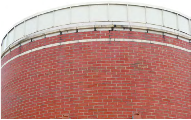
46. Exterior - Moisture staining along concrete details at middle school entry
