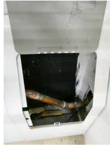
106. MEP - Copper piping for hydronic system
