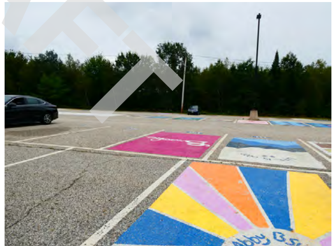
4. Site - North parking surface condition
