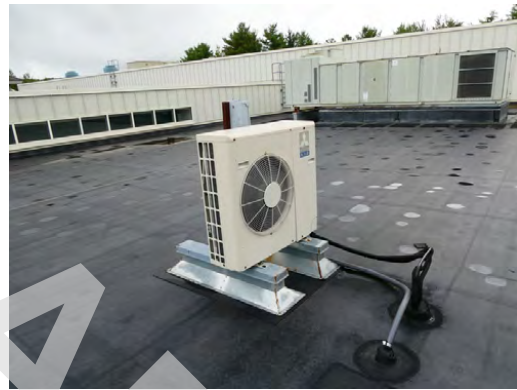
MEP - Older roof mounted heat pump for ductless system
