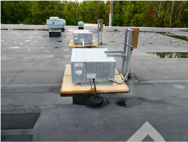
117. MEP - Kitchen refrigeration condensers
