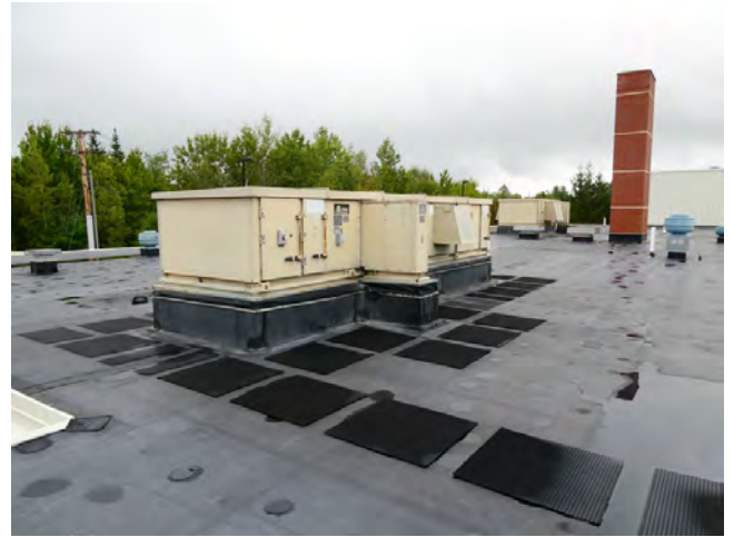
118. MEP - Packaged roof top unit
