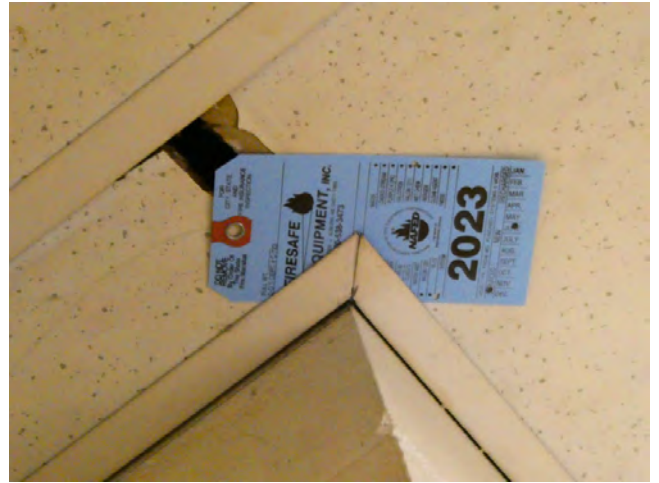
142. FLS - ANSUL fire suppression system concealed in ceiling
