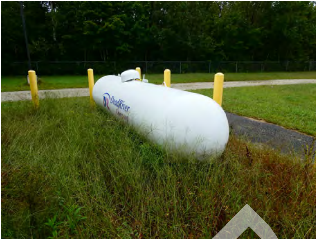
109. MEP - Onsite propane tank for fuel
