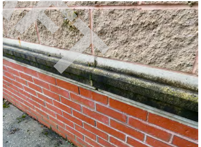
52. Exterior - Moisture staining along concrete band (courtyard)
