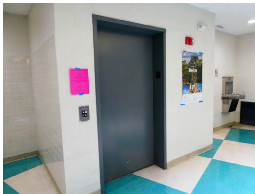
Vertical Transportation - Elevator for the high school area
