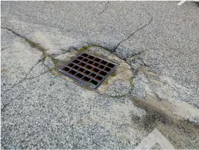
9. Site - Asphalt pavement condition at north parking area
