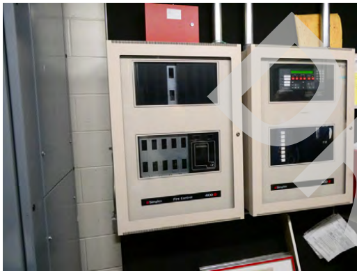
FLS - Main fire alarm control panels
