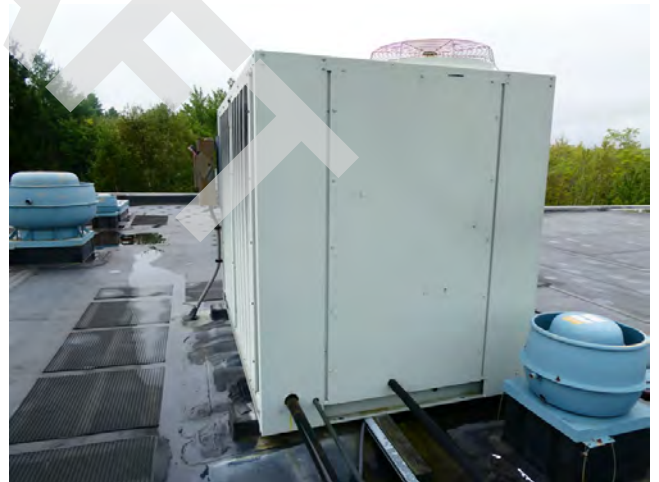
124. MEP - Roof mounted air cooled packaged chiller
