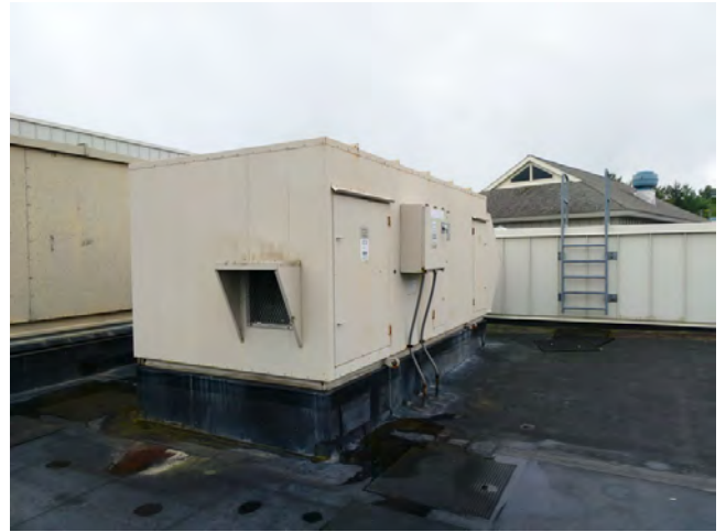
122. MEP - Roof mounted air recovery unit
