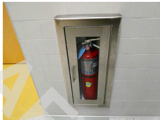
FLS - Cabinet mounted fire extinguishers in common areas
