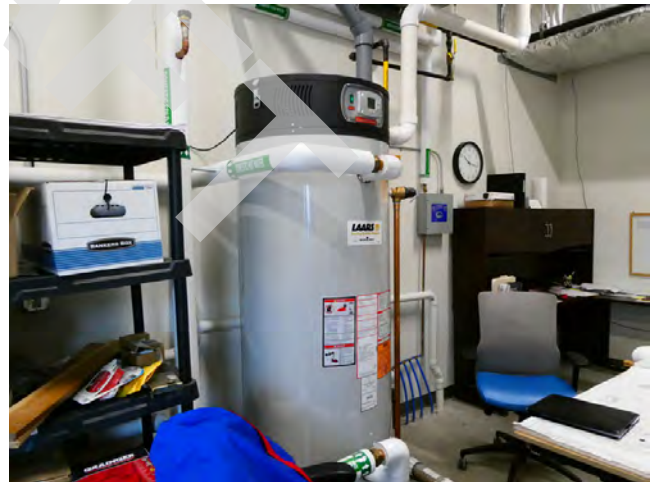
104. MEP - Propane sourced domestic water heater for middle school
