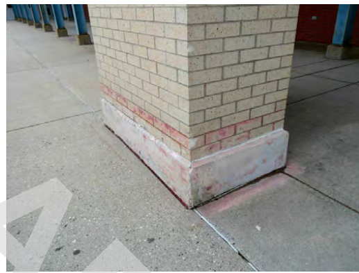
Exterior - Deteriorated EIFS at base of columns (main entrance)
