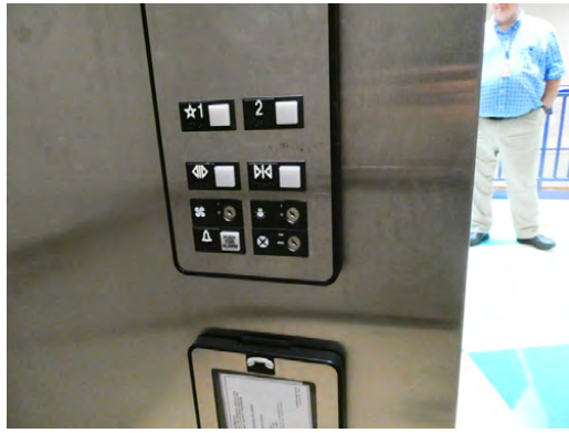
Vertical Transportation - Elevator controls
