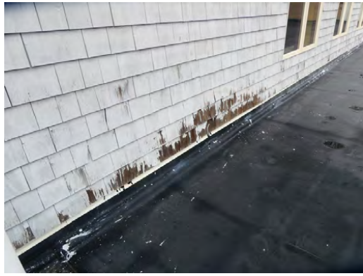
Exterior - Deteriorated stain finish at wood siding
