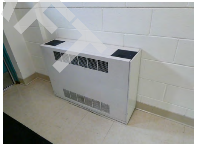
128. MEP - Wall mounted cabinet forced air units
