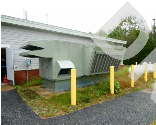
MEP - Packaged outdoor air unit for the middle school common areas
