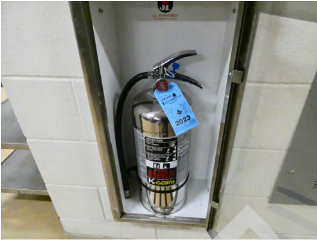
145. FLS - Chemical extinguisher in the commercial kitchen area
