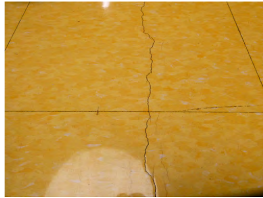
Interiors - Isolated areas of stress cracking at common area vinyl flooring
