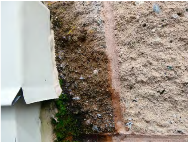
51. Exterior - Moisture staining at east elevation (roofline)
