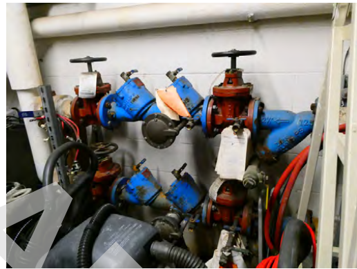
MEP - Backflow preventer in mechanical room
