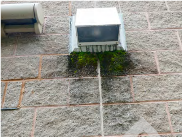
49. Exterior - Moisture staining and organic growth along CMU (courtyard)
