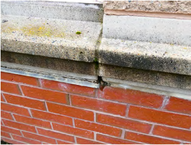
47. Exterior - Moisture staining along concrete window sill (courtyard)
