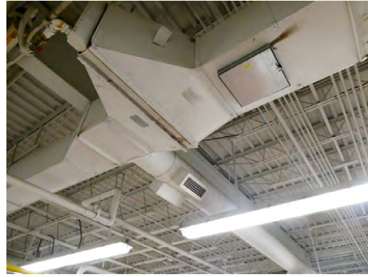
MEP - Middle school gymnasium ducting system
