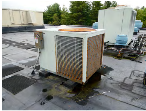
MEP - Older roof mounted air cooled condenser
