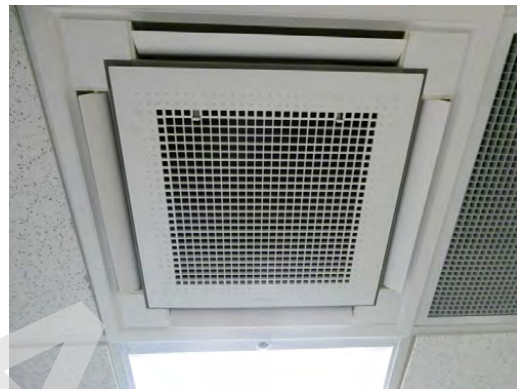
MEP - Ceiling mounted VRV indoor unit
