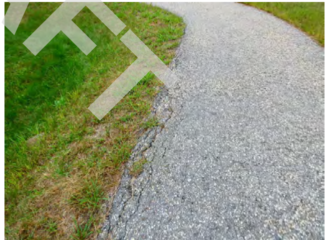
8. Site - Deterioration along asphalt paved walkway
