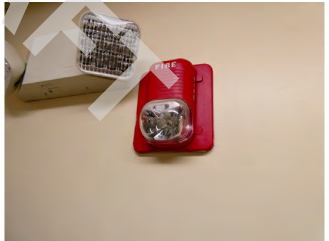
36. FLS - Emergency strobe lighting
