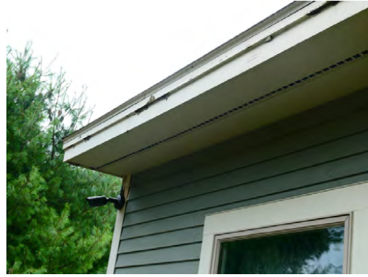
Exterior - Worn paint finish at fascia board
