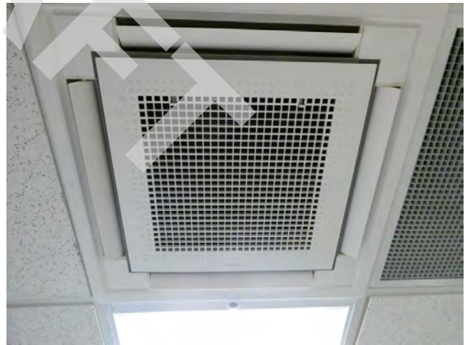
28. MEP - Ceiling mounted VRV indoor unit
