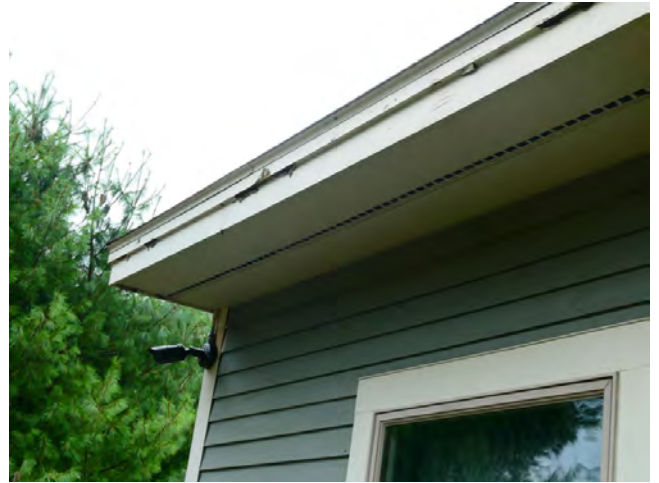
22. Exterior - Worn paint finish at fascia board
