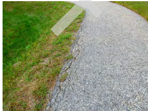
Site - Deterioration along asphalt paved walkway
