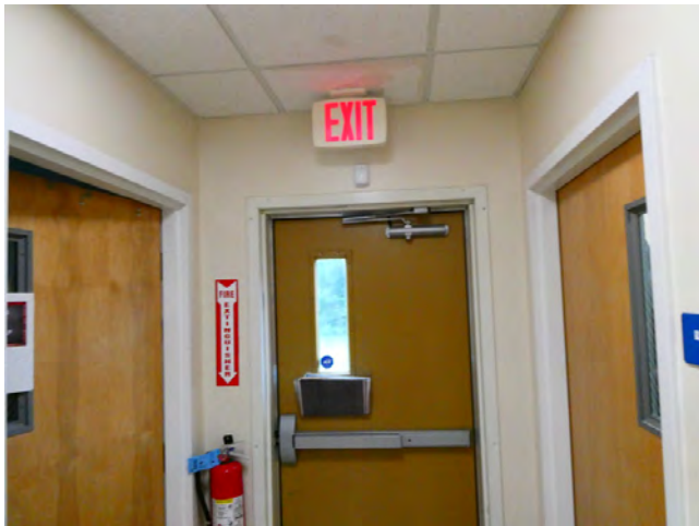
39. FLS - Lighted emergency exit signage
