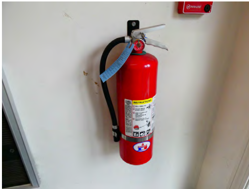
FLS - Wall mounted fire extinguishers
