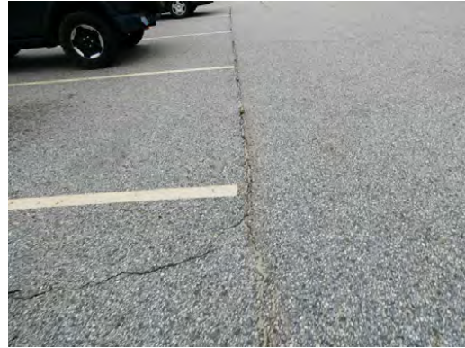
Site - Isolated longitudinal cracking along south parking area
