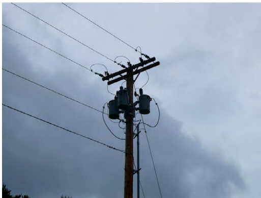
MEP - Pole mounted electrical transformer
