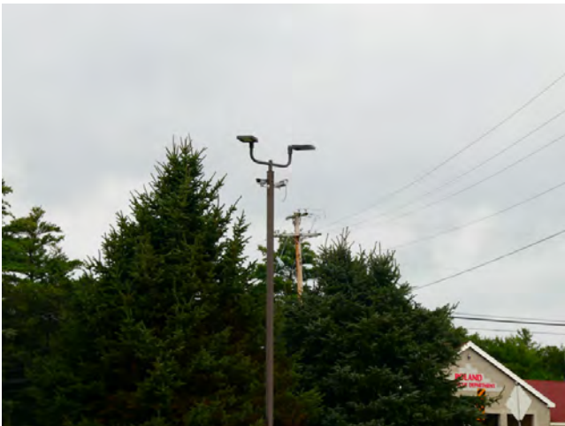
11. Site - Pole mounted light fixtures at parking area perimeter
