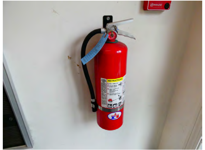
34. FLS - Wall mounted fire extinguishers
