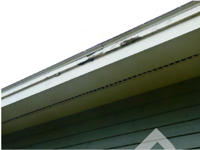
21. Exterior - Worn paint finish at fascia board
