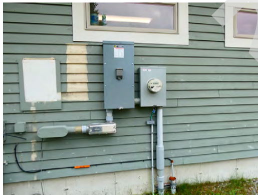
MEP - Main service panel along west elevation
