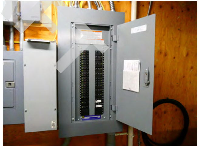
32. MEP - Main electrical panel
