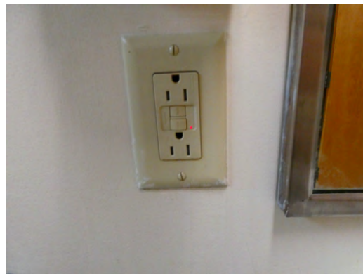
MEP - GFCI outlet in toilet room
