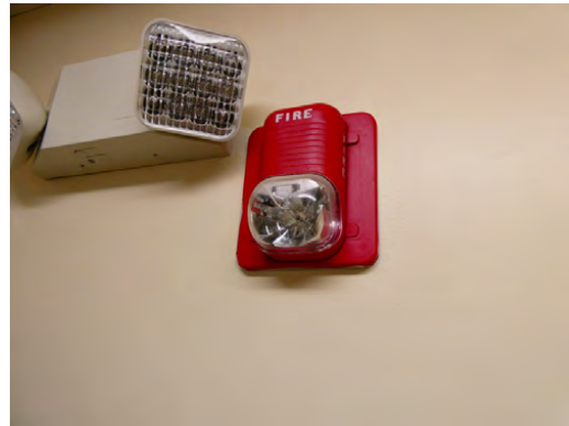
FLS - Emergency strobe lighting
