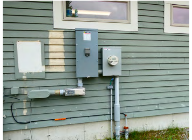
30. MEP - Main service panel along west elevation
