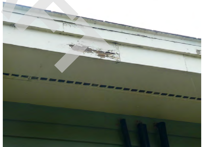
20. Exterior - Worn paint finish at fascia board
