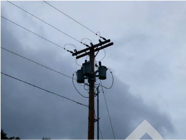
29. MEP - Pole mounted electrical transformer
