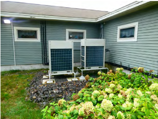
27. MEP - VRV exterior units
