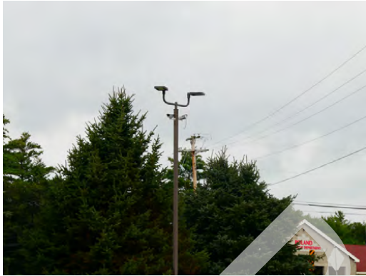
Site - Pole mounted light fixtures at parking area perimeter
