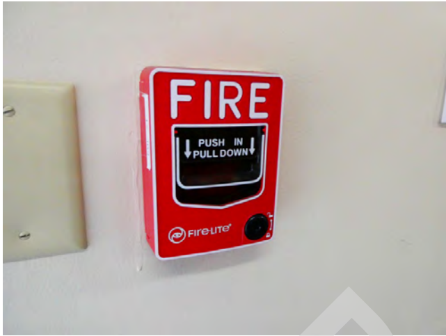
37. FLS - Fire pull stations in common corridors
