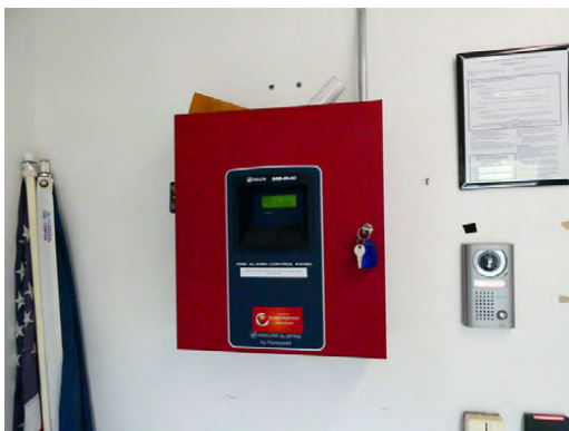
FLS - Main fire alarm control panel
