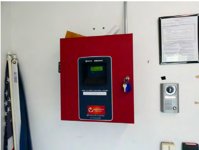
35. FLS - Main fire alarm control panel
