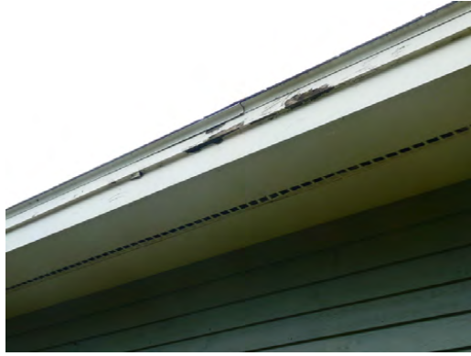
Exterior - Worn paint finish at fascia board
