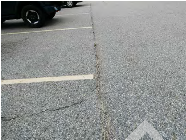
5. Site - Isolated longitudinal cracking along south parking area
