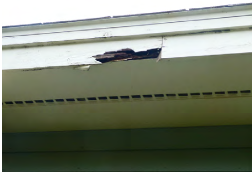
Exterior - Sectional deterioration at fascia board
