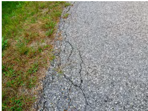
Site - Deterioration along asphalt paved walkway
