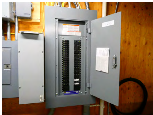
MEP - Main electrical panel
