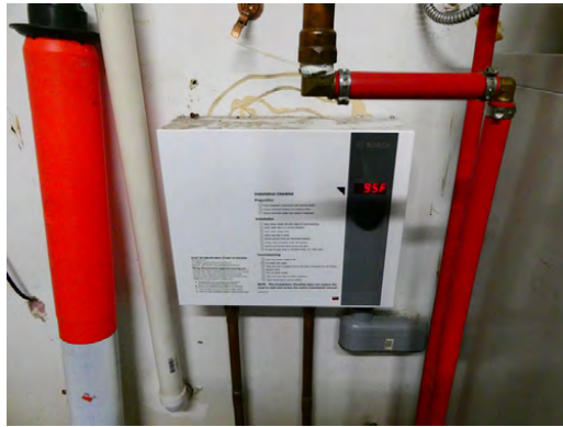
MEP - Electric tankless water heater
