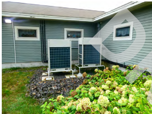
MEP - VRV exterior units
