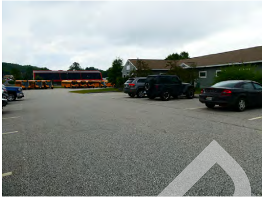
Site - South parking area and pavement condition
