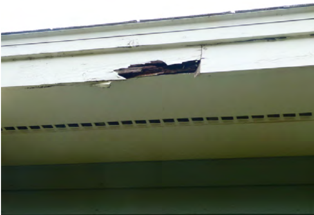
19. Exterior - Sectional deterioration at fascia board
