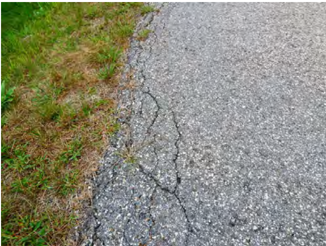
7. Site - Deterioration along asphalt paved walkway
